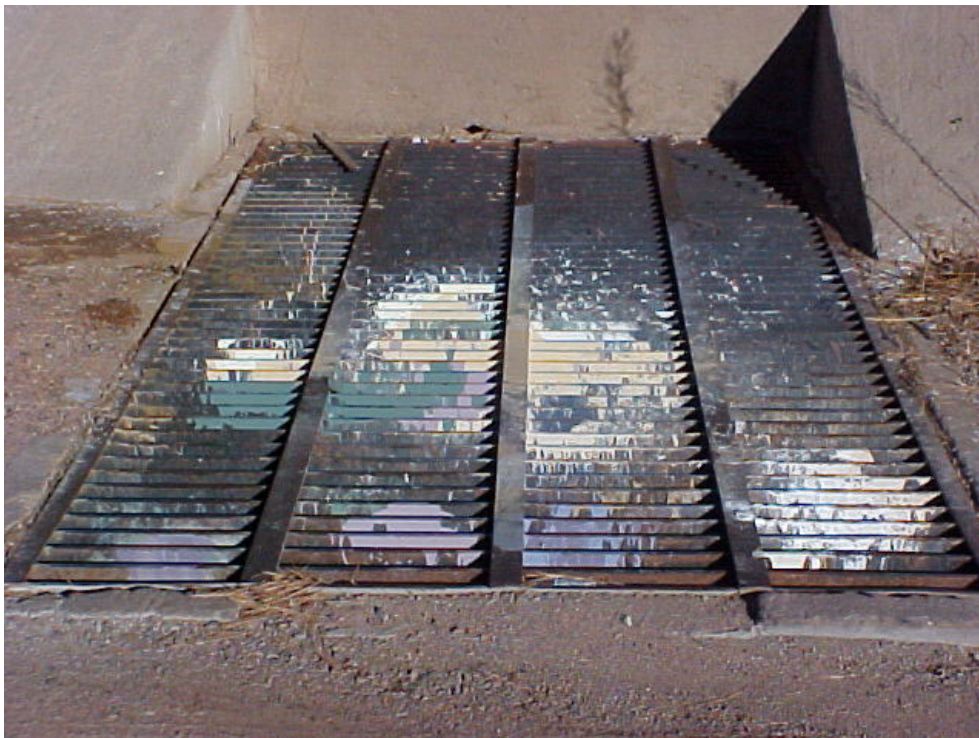
Paint and chemicals that were drained into a storm drain.
