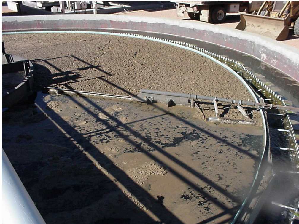
Primary Wastewater Treatment Clarifier.
