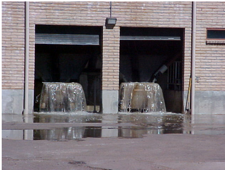
Headworks flooding or overflowing because of high grease loading.
