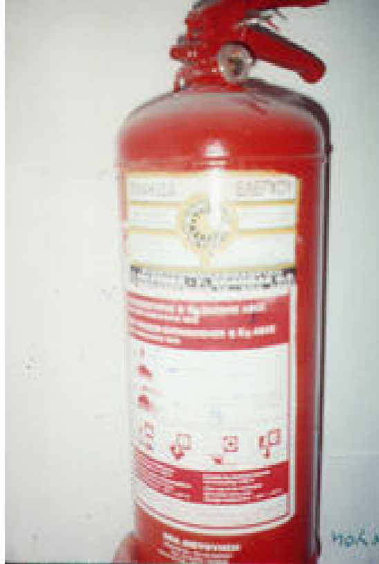
Fire Extinguisher without a discharge hose, a disaster waiting to happen.
