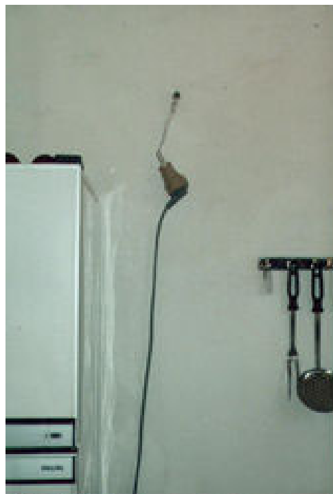
Dangerous electrical wiring, fire waiting to happen.
