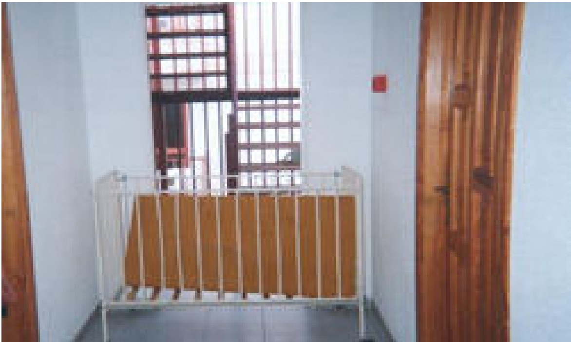
Blocked Fire Exit. Death trap.
