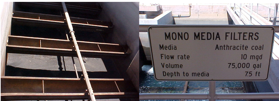
Dried backwash channels on the top of a cleaned filter bed.
