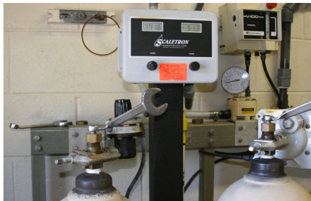
150-pound chlorine gas cylinders on a scale and in service.
