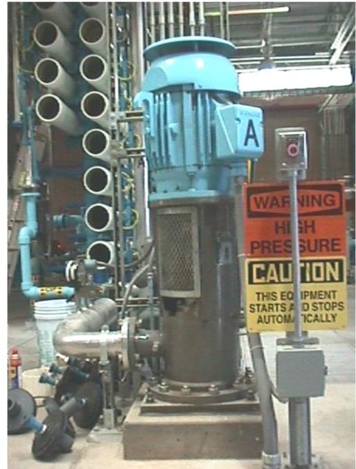
Membrane Filtration System
