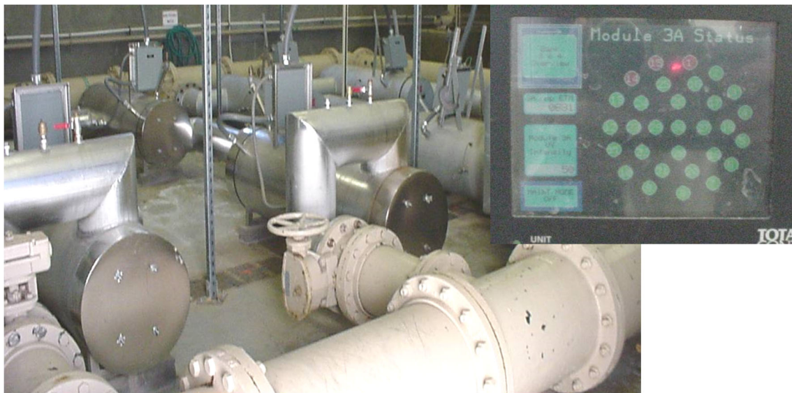
UV Trains and SCADA display.
