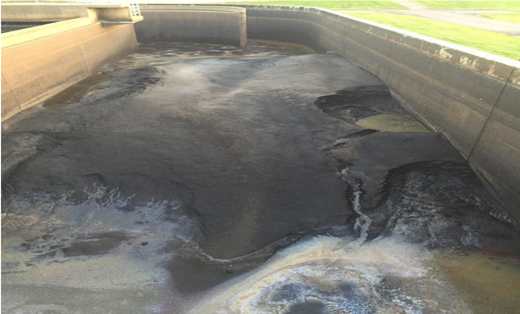
The results of not having grit removal. Filling part of an oxidation ditch aeration tank.
