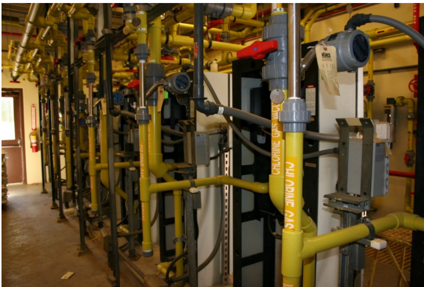
Chlorine Gas Feed Room
