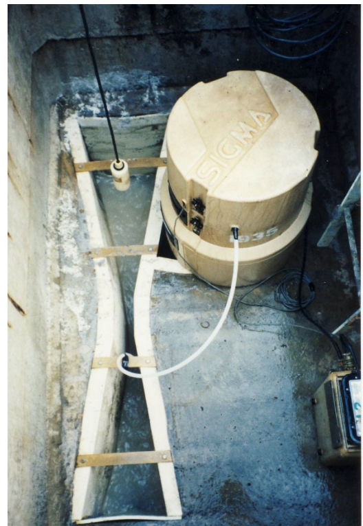
Automatic sampler inside a vault.
