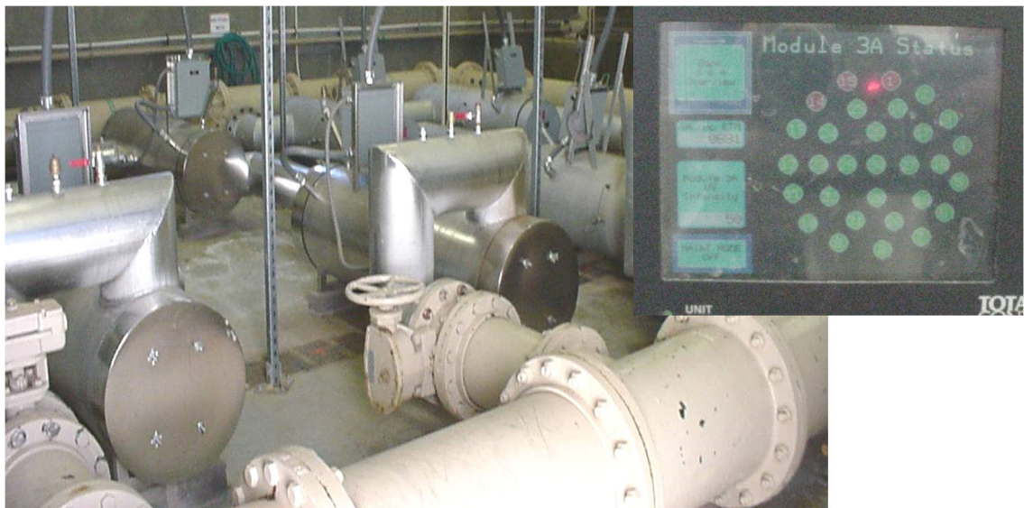
UV Trains and SCADA display.
