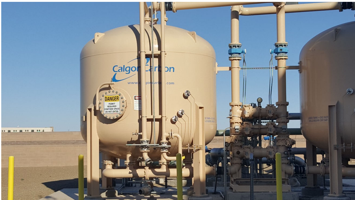
Granular Activated Carbon (GAC) vessel
