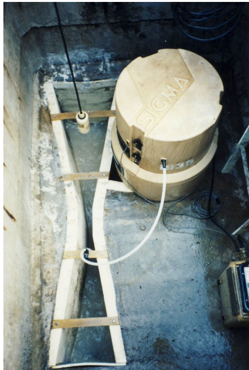
Automatic sampler inside a vault.
