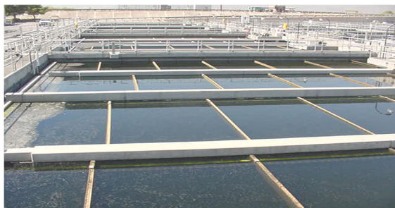
Rectangular Secondary Clarifier
