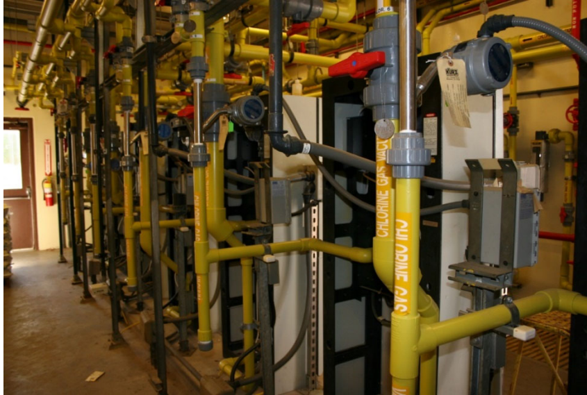
Chlorine Gas Feed Room
