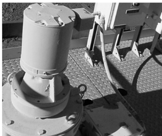
Clarifier Drive Motor
