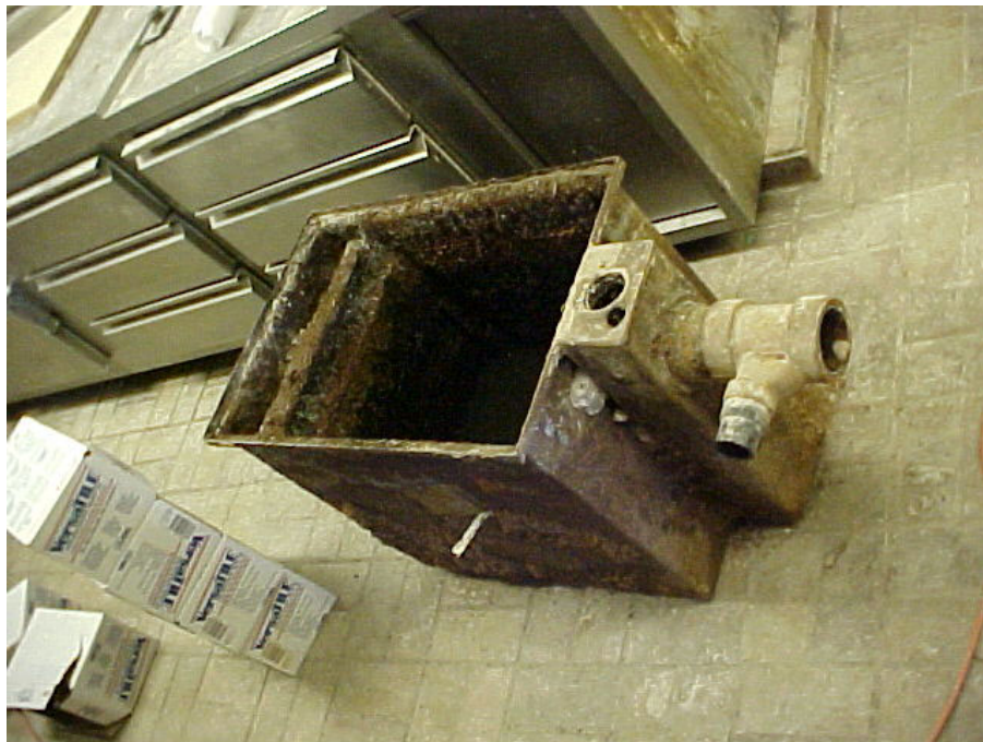
In-floor Grease trap being removed and replaced with a grease interceptor. Unfortunately, most grease traps are not properly maintained.
