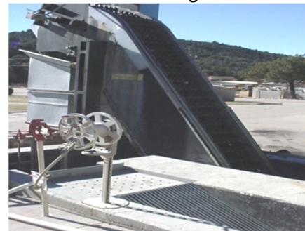
Manual and Mechanical Bar Screens
