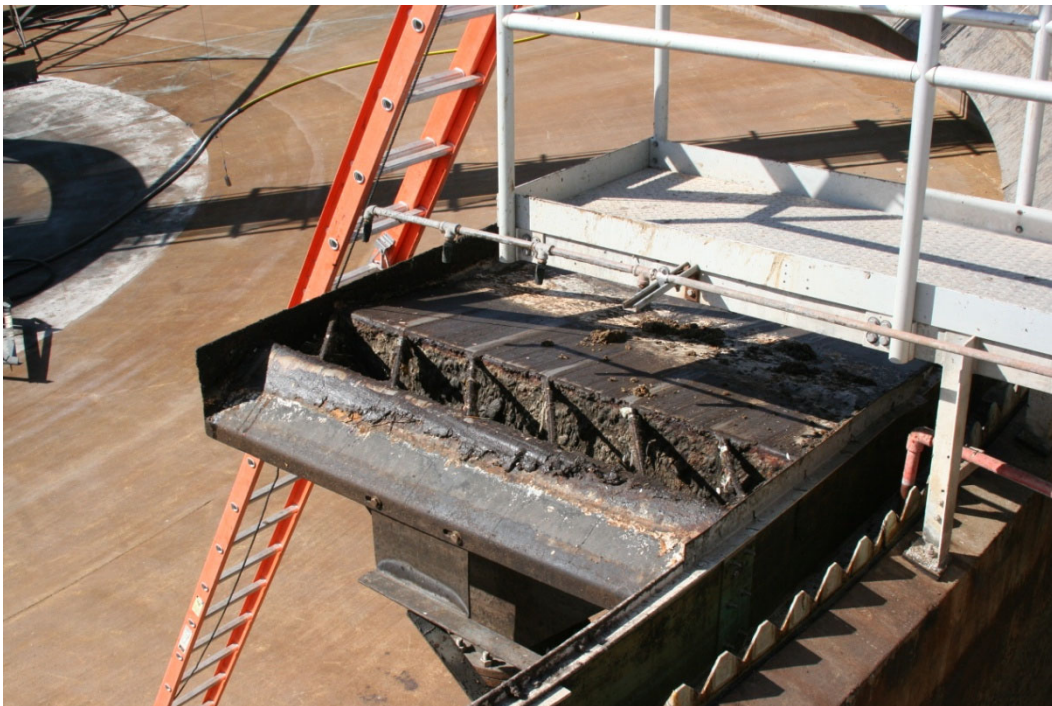
Scum Box located on a circular clarifier.
