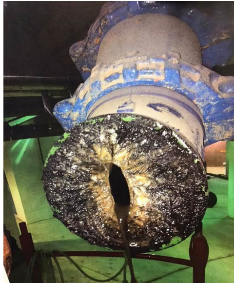
Struvite deposits inside a digester pipe.
