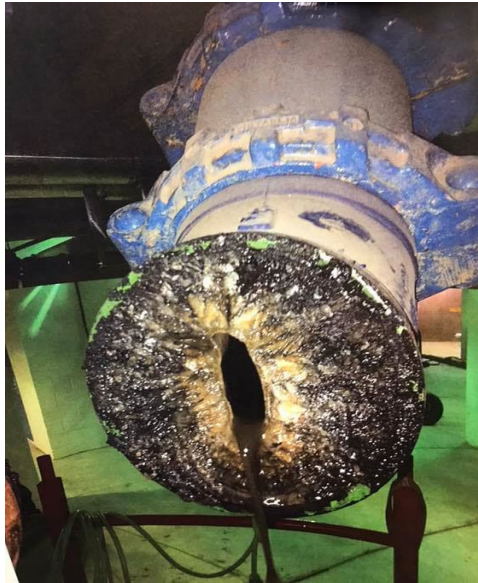
Struvite deposits inside a digester pipe.
