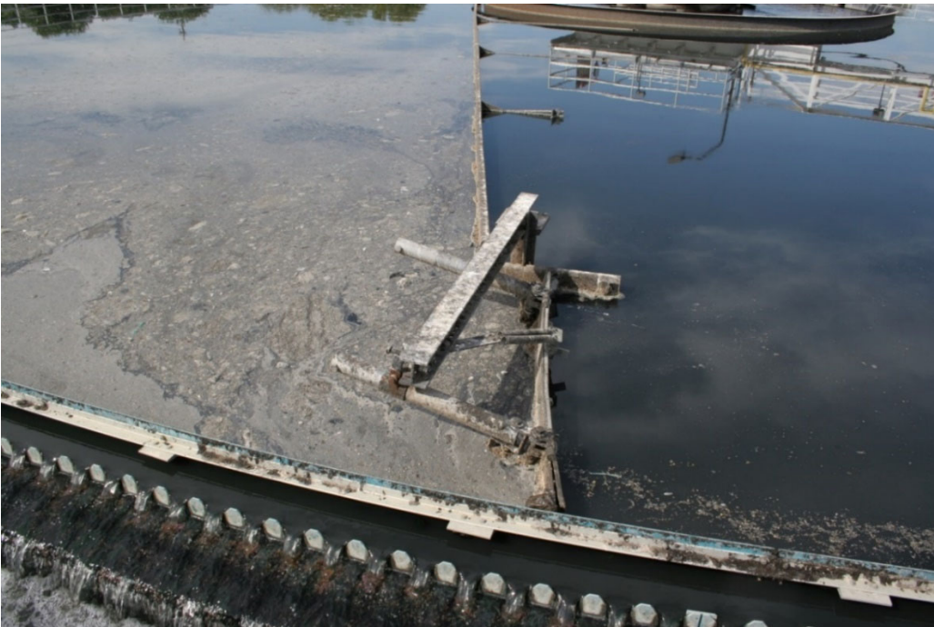
Bottom, scum armature skimmer on a secondary clarifier.
