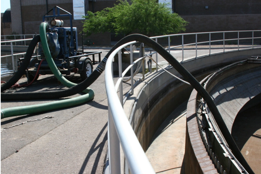
This circular clarifier has been dewatered with a portable pump Maintenance on a circular clarifier should be performed annually.
