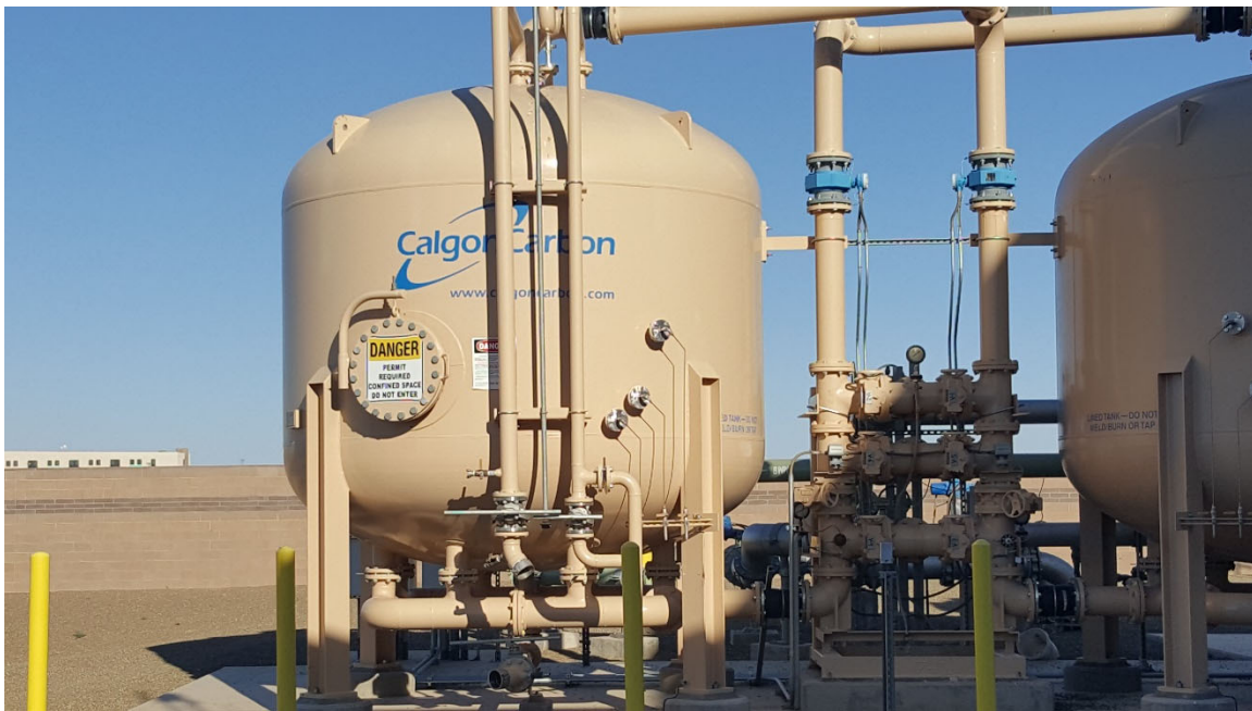
Granular Activated Carbon (GAC) vessel
