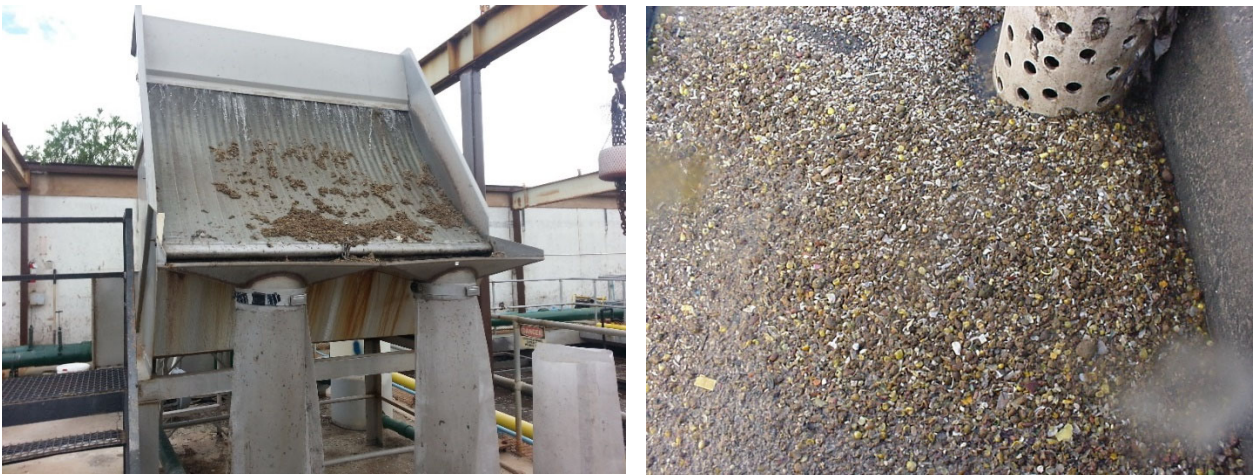
Left, Strainer Screen, Right, Floating debris in an influent wetwell
