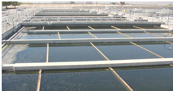
Rectangular Secondary Clarifier
