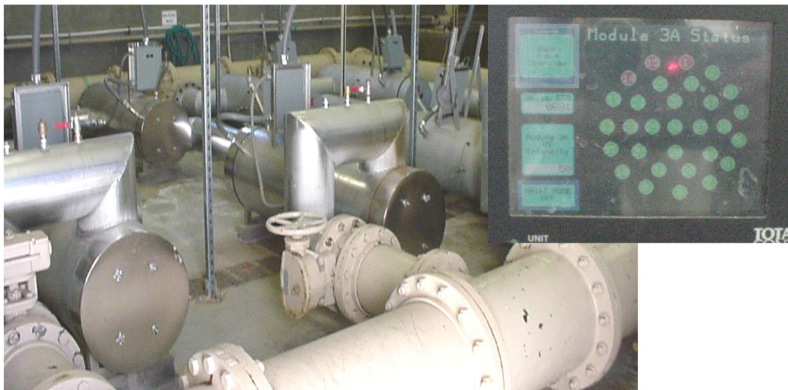
UV Trains and SCADA display.
