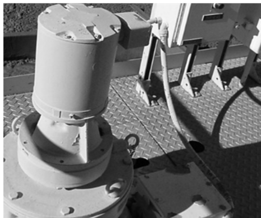
Clarifier Drive Motor
