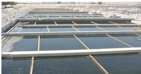
Rectangular Secondary Clarifier
