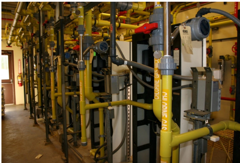
Chlorine Gas Feed Room
