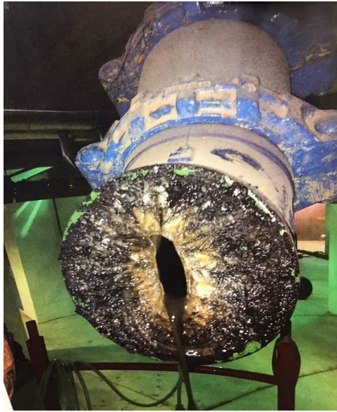
Struvite deposits inside a digester pipe.
