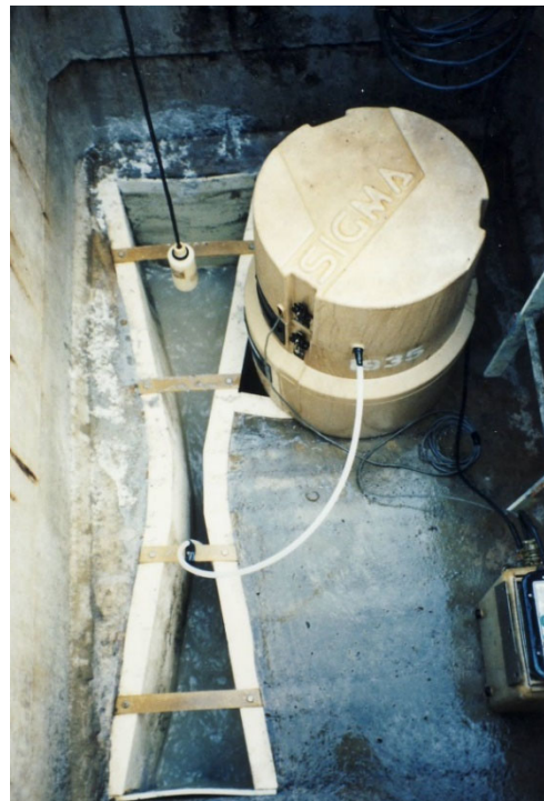
Automatic sampler inside a vault.
