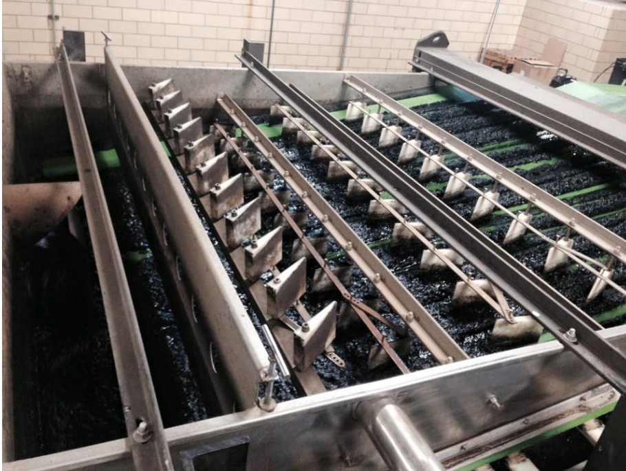
Example of a Sludge Press.
