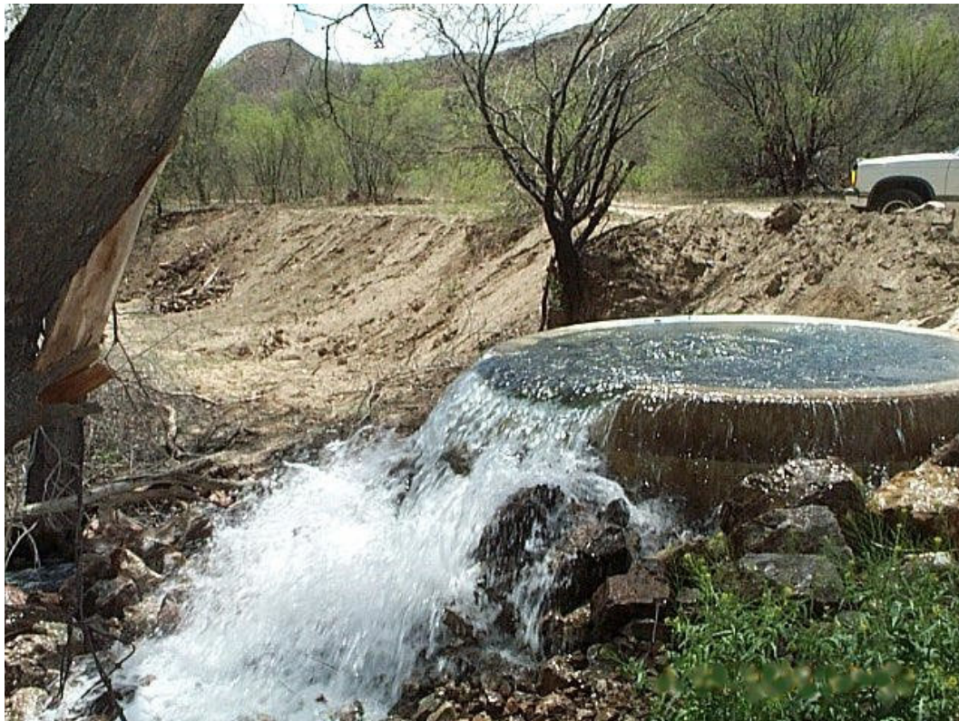
Treated wastewater outfall.
