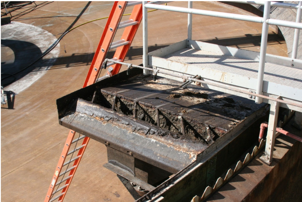
Scum Box located on a circular clarifier.
