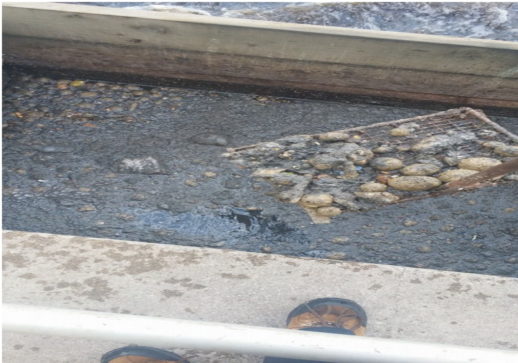
A buildup of grease balls in an oxidation ditch.
