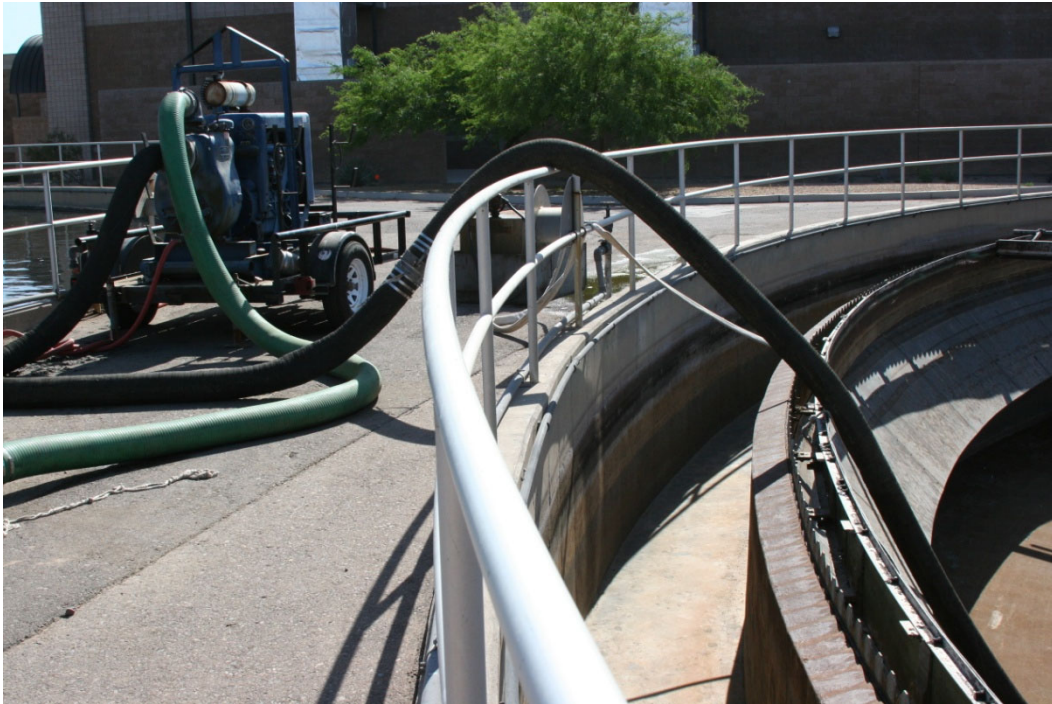
This circular clarifier has been dewatered with a portable pump Maintenance on a circular clarifier should be performed annually.
