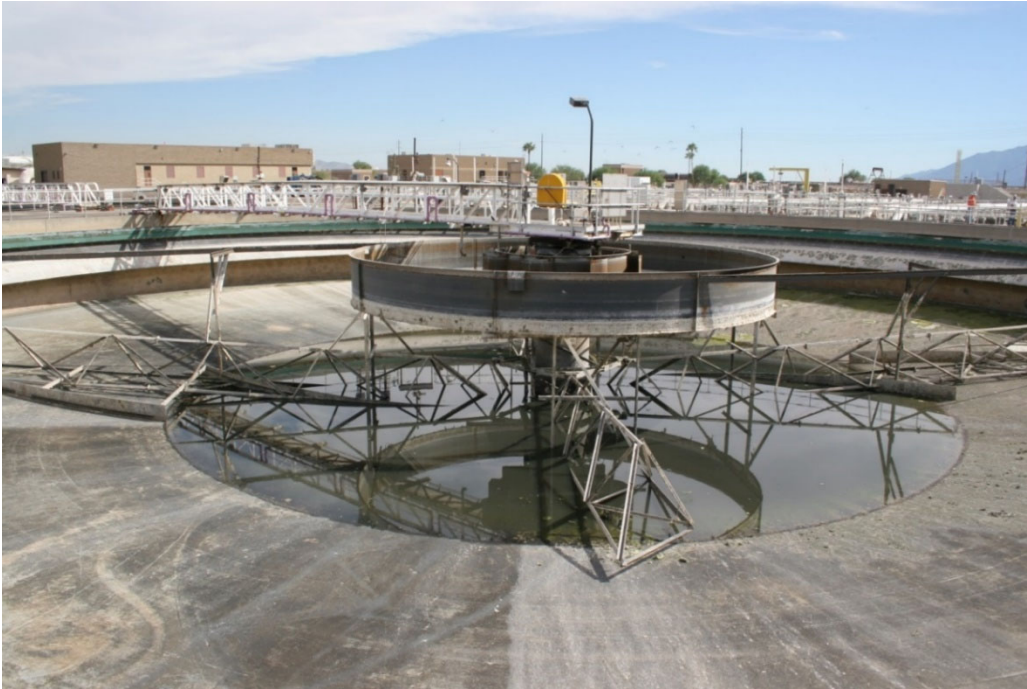
Top photograph, a clarifier's raking mechanism.
