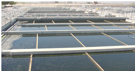
Rectangular Secondary Clarifier
