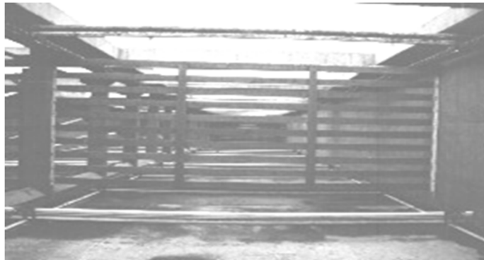
Baffles to dissipate flow in a rectangular secondary clarifier.
