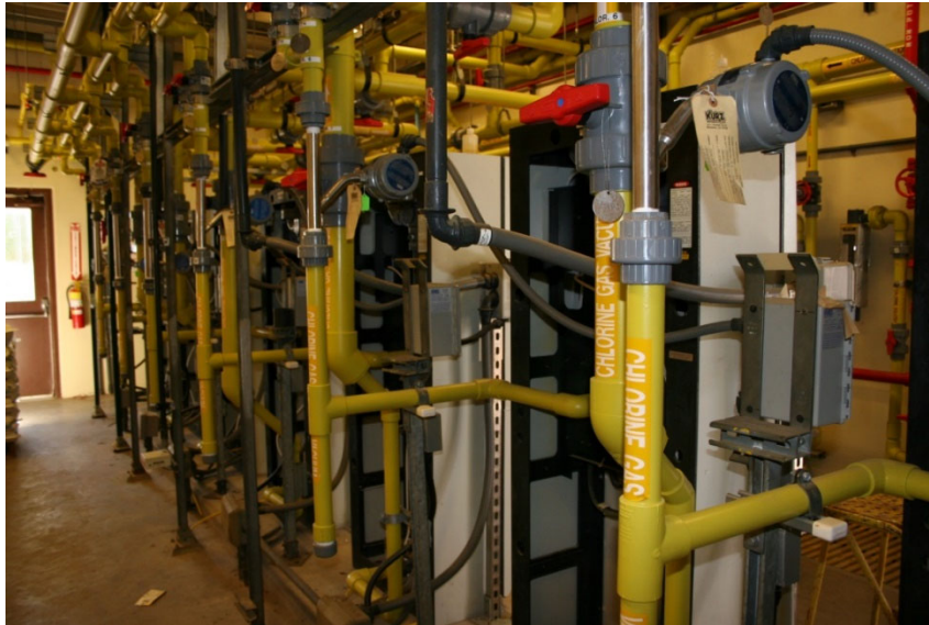
Chlorine Gas Feed Room
