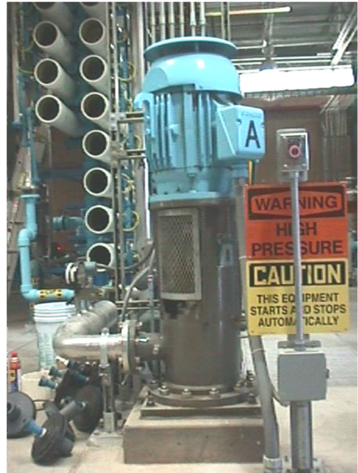
Membrane Filtration System
