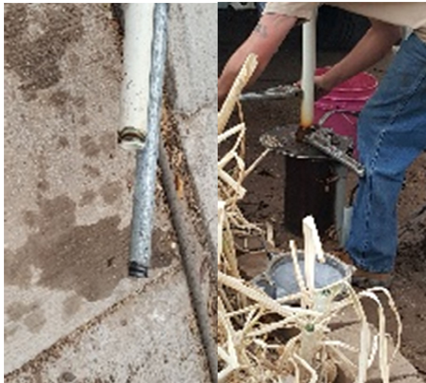
Attachment that screws into well pipe to be pulled. Metal disk supports couplings on wellhead while being pulled.
