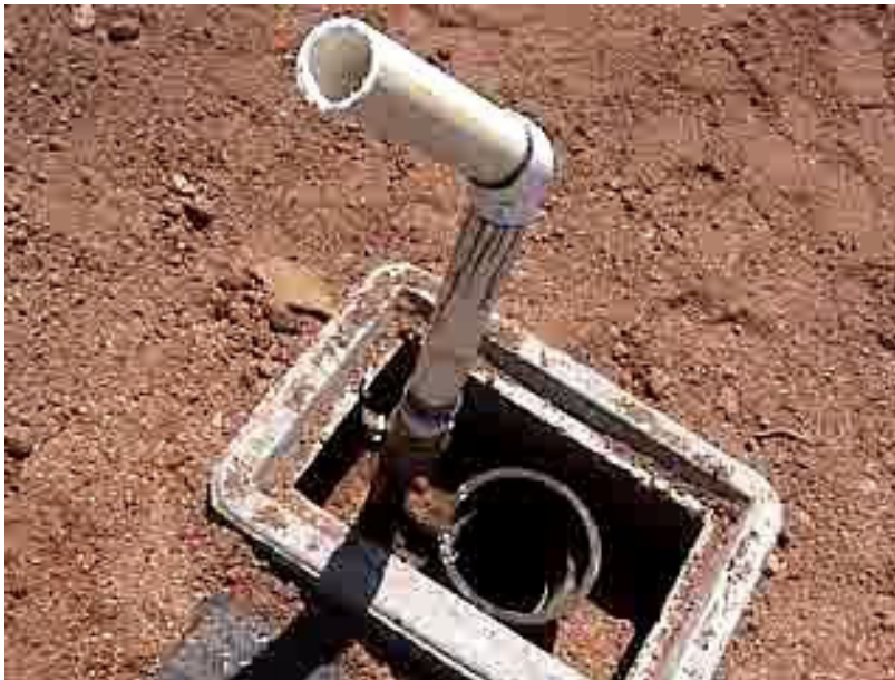
A temporary blow-off at a dead-end line.
