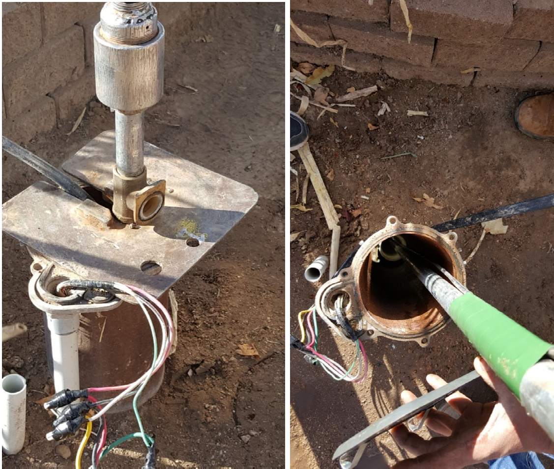
The discharge side of the pipe has a tee that seats on a saddle down below ground to prevent freezing.
