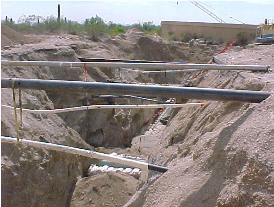
Supporting utilities is mandatory.
