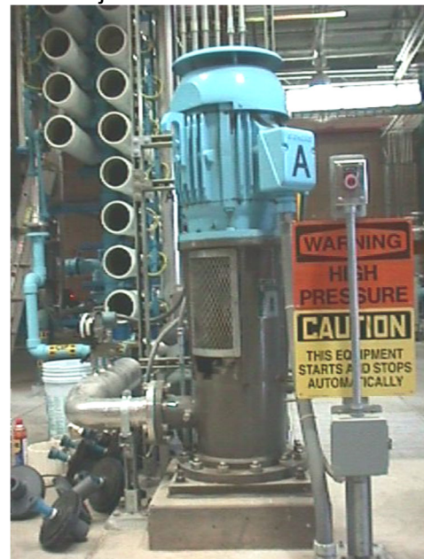
Membrane Filtration System
