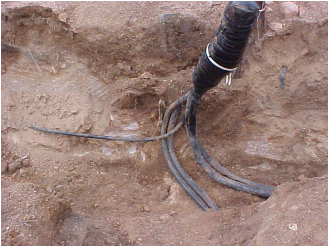
Telephone Cables, nasty to dig around. It's almost as bad as electric lines.
