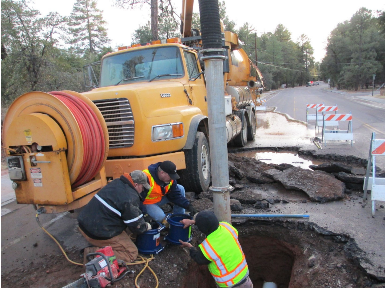
A normal day of work for most distribution system operators. Using a Vector to pump out the hole while replacing a plastic main section.
