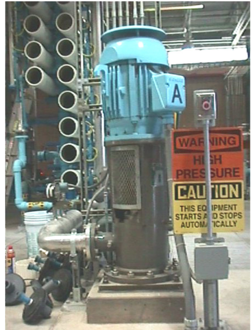
Membrane Filtration System
