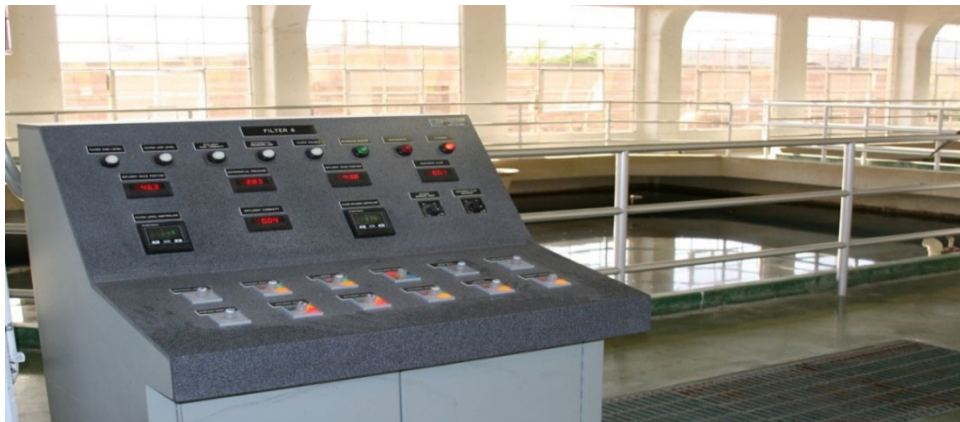
A filter control panel.
