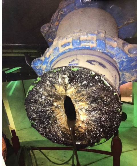
Struvite deposits inside a digester pipe.
