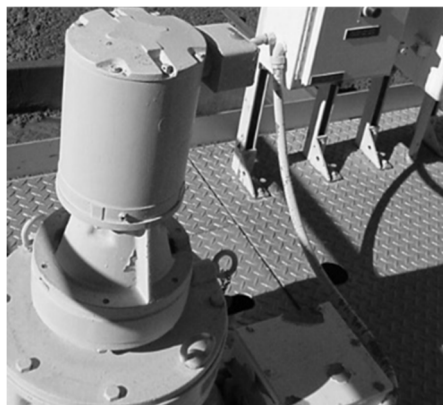
Clarifier Drive Motor
