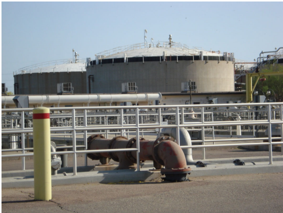
These two above ground circular tanks are massive anaerobic digesters.
