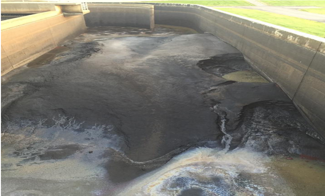
The results of not having grit removal. Filling part of an oxidation ditch aeration tank.
