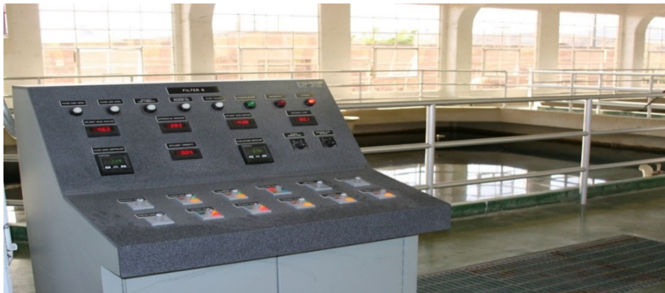
A filter control panel.
