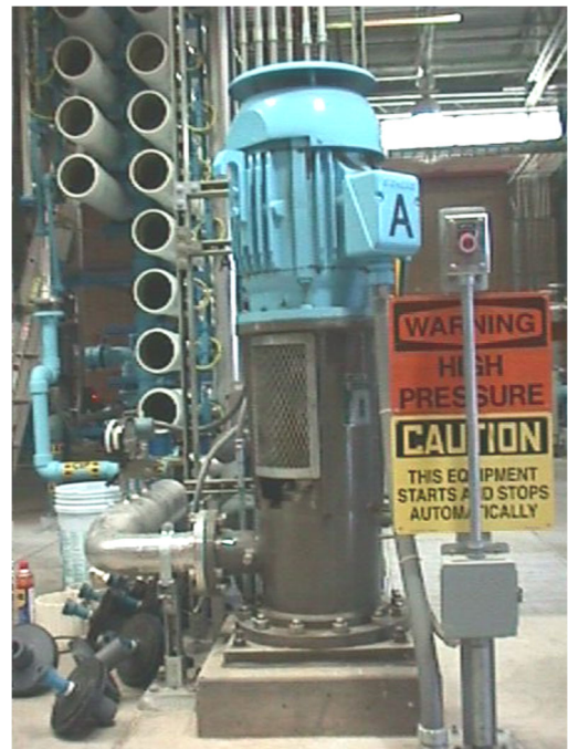
Membrane Filtration System
