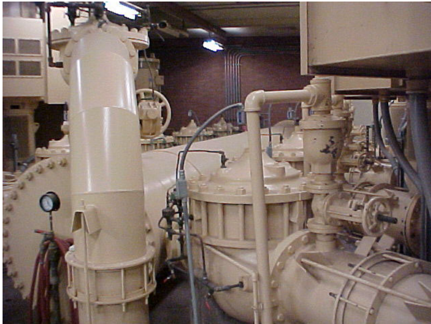
Inside a giant booster pump station.
