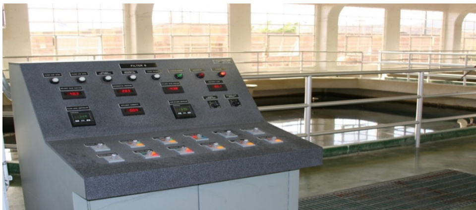
A filter control panel.
