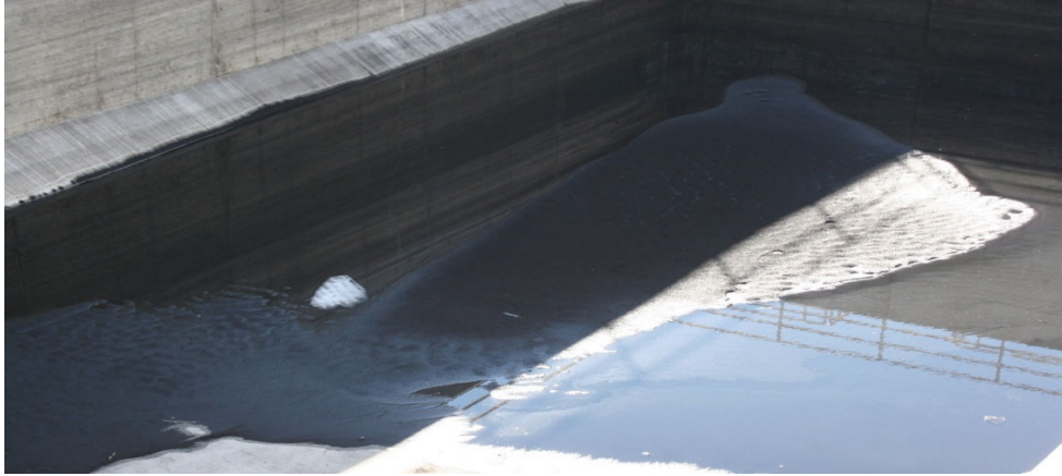
A backwash basin that has wasted or lost media caked on the bottom.
