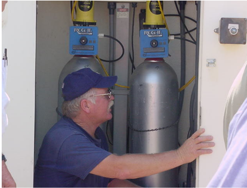
150-Pound Chlorine Cylinder
