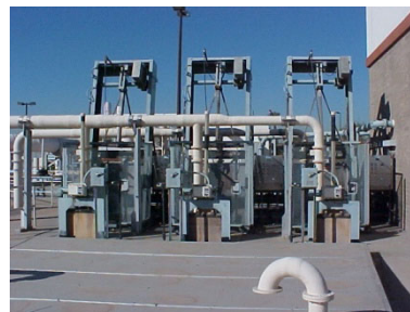
Wastewater Headworks In the top 10 Vulnerable Terrorist Targets, easy to destroy and able to cause mass disease.
