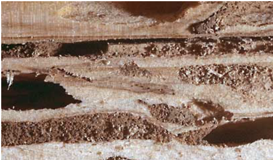
Termite gallery structure or what humans call “serious home damage”.
