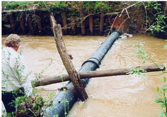
Downstream of a nonfunctional Combined Sewer Overflow (CSO) Control Facility.
