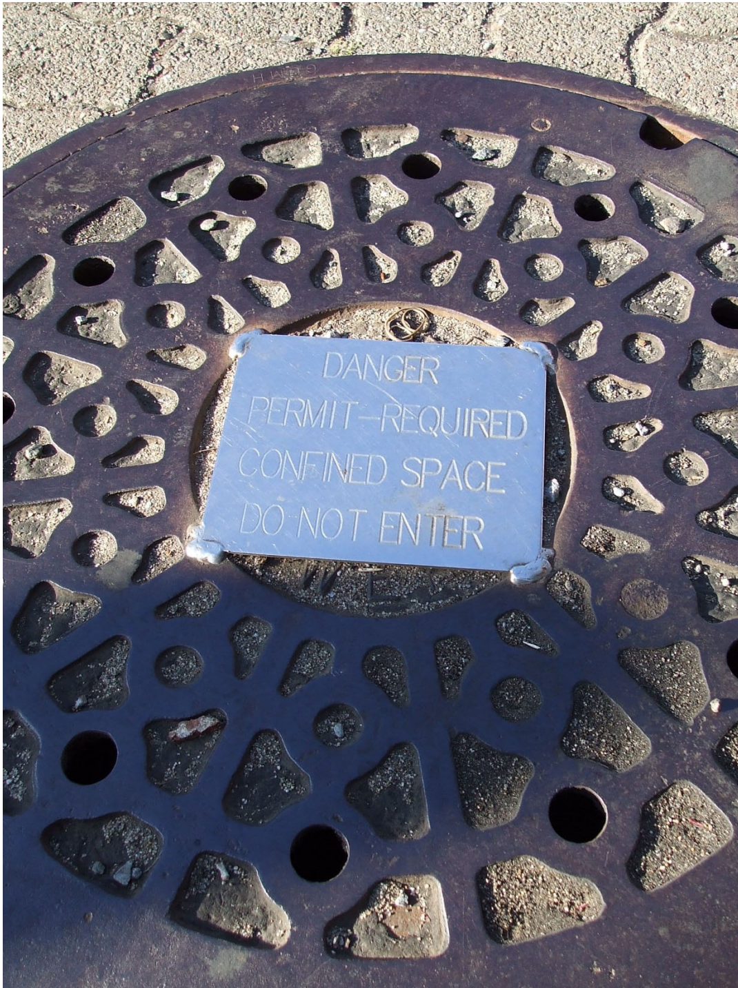
A great method of attaching permit-required signage to a storm drain cover. Again, found throughout San Francisco.
