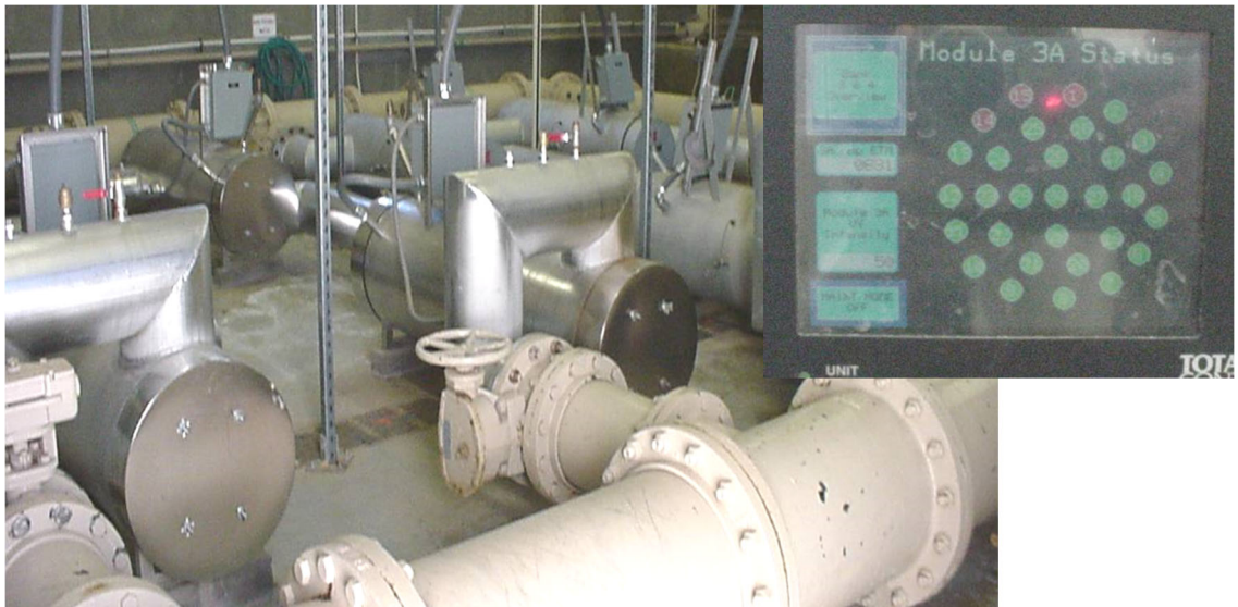
UV Trains and SCADA display.
