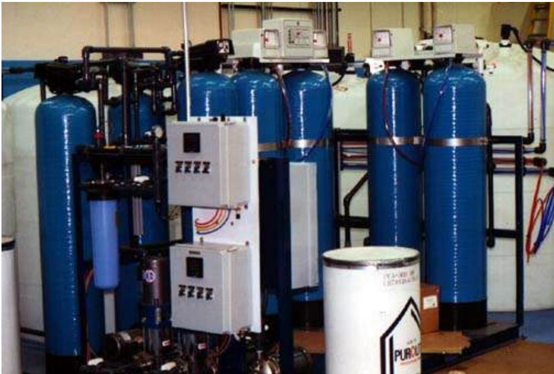
Ion Exchange Units
