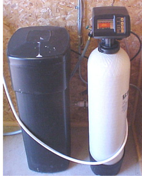
Softener with brine tank on right
