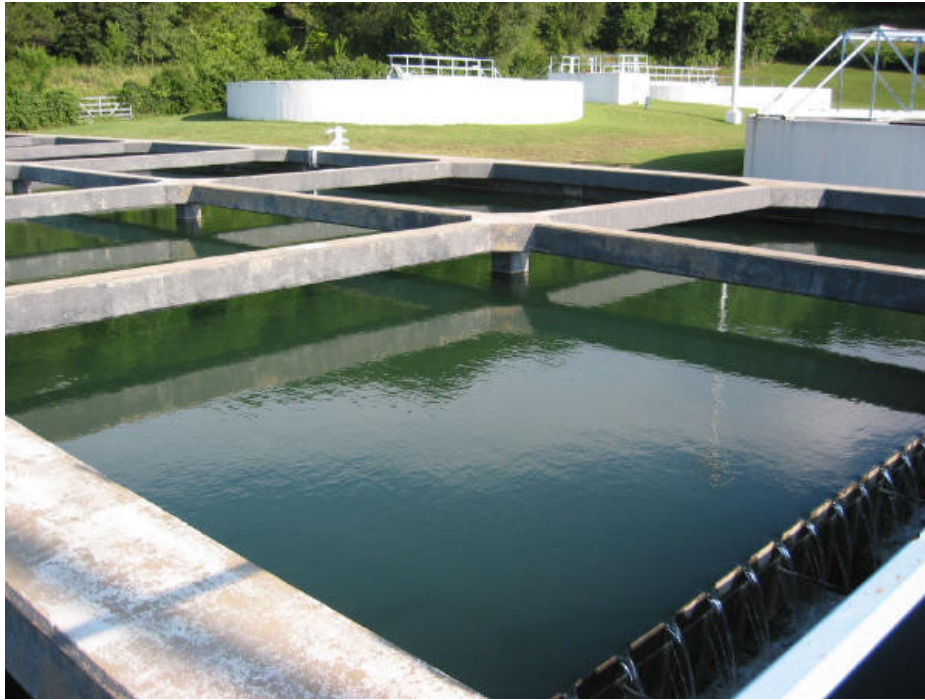
Top Photograph - Final Rectangular Sedimentation Basin Discharge Weirs
