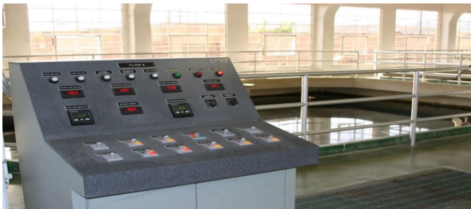
A filter control panel.
