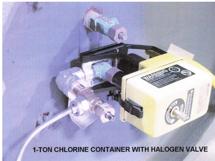
1-TON CHLORINE CONTAINER VALVES
