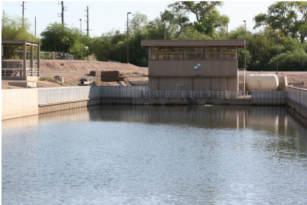
Raw Water Intake Requires corrosion protection
