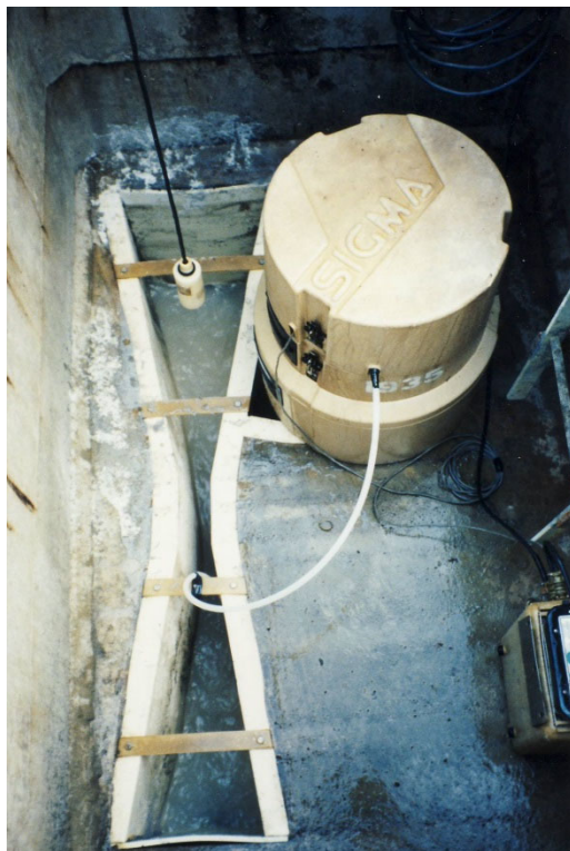
An automatic programmable wastewater sampler inside a customer's vault.
