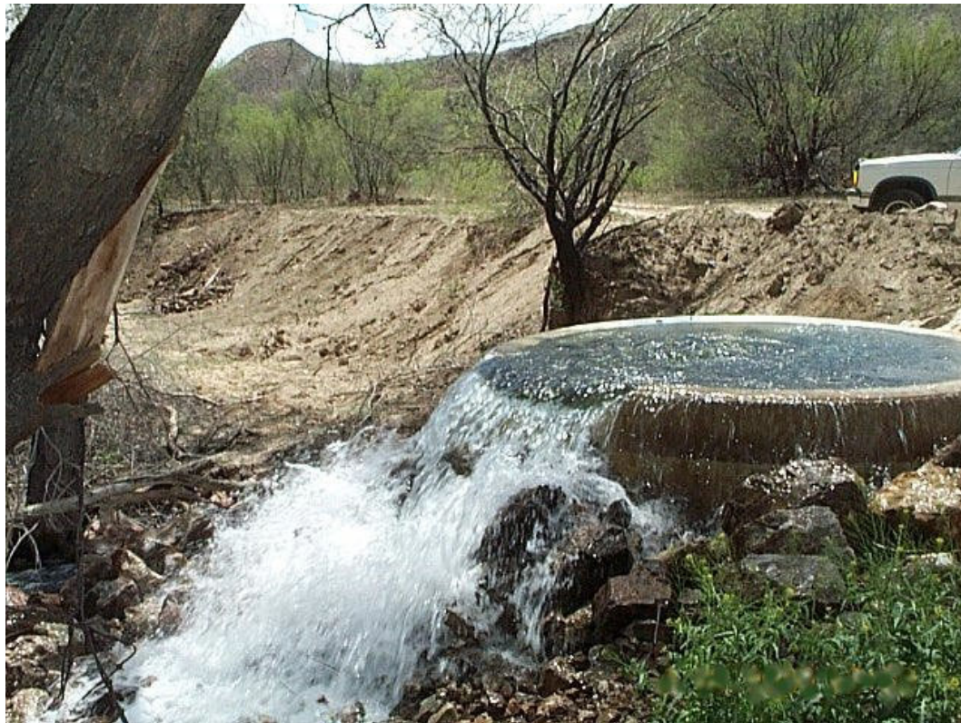
Treated wastewater outfall.
