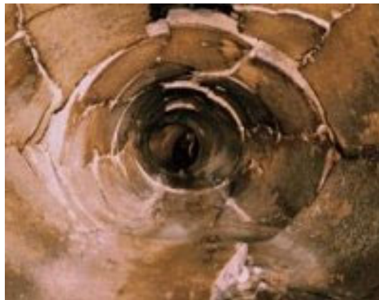
Above, a cracked sewer main, a SSO waiting to happen.
