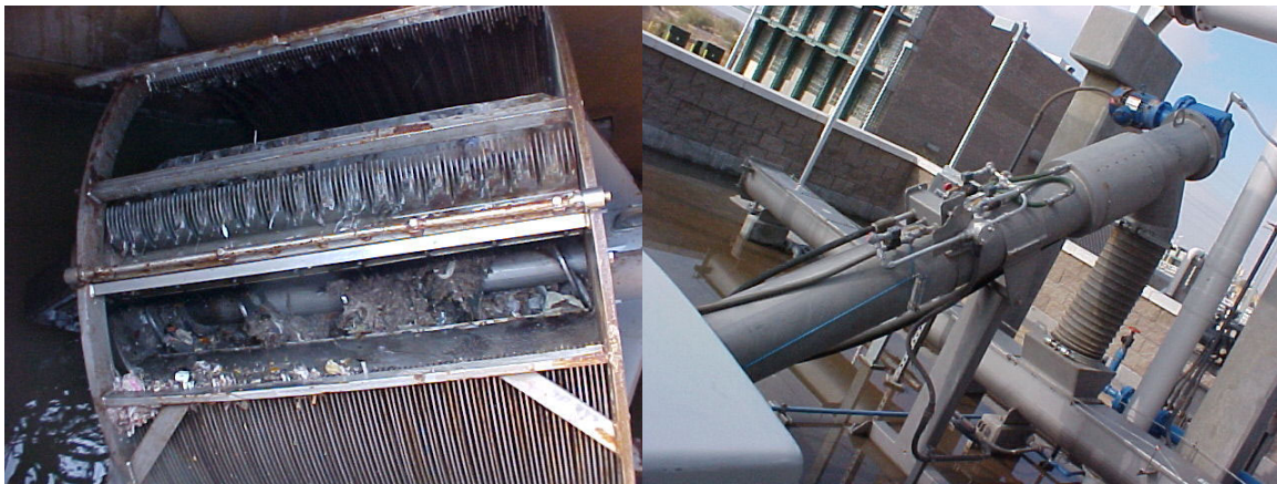
Headworks' Rotating Bar screen and screening handling.
