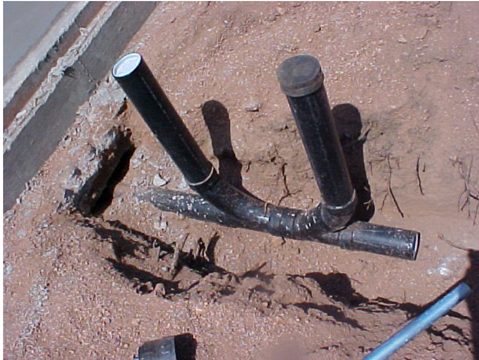
2-Way Cleanout DWV Soil Pipe, needs to be within 2 feet of the house, perpendicular (not parallel) to the footing and the end or grade level needs to be painted to protect from sunlight.
