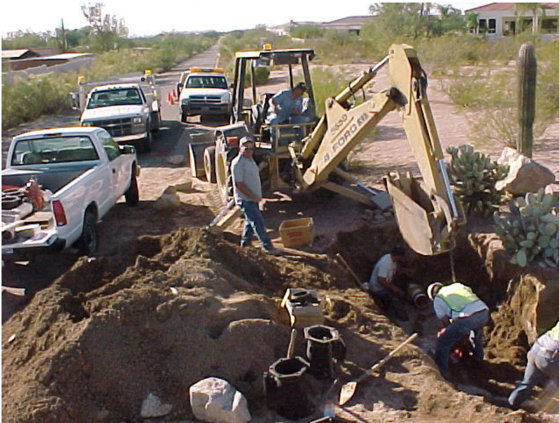
Repair crew replacing three tapping valves that blew out during a leak.
