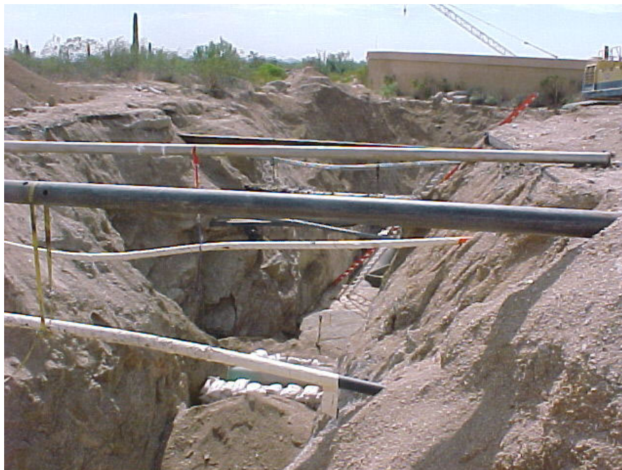
Supporting utilities is mandatory.
