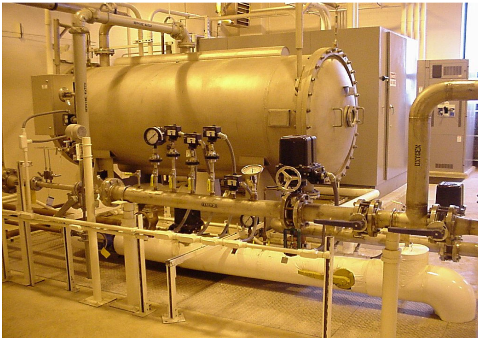
Large Ozone generator
