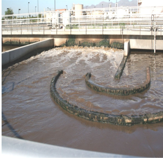
Oxidation ditch baffles slowing down the flow.
