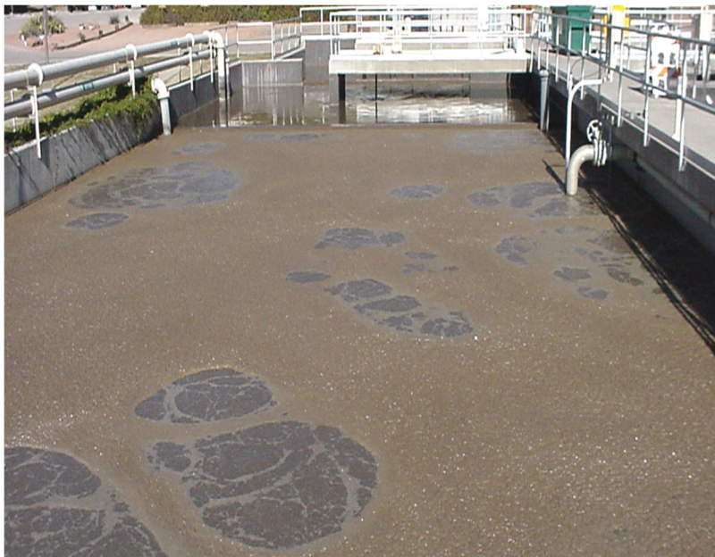
Activated Sludge Aeration Basin, identified by the bubbles.
