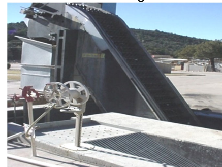
Manual and Mechanical Bar Screens
