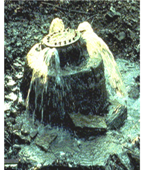
Sanitary Sewer Overflow
