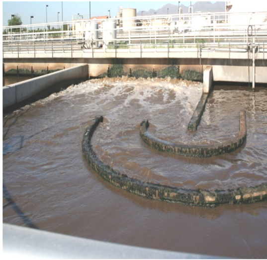
Oxidation ditch baffles slowing down the flow.
