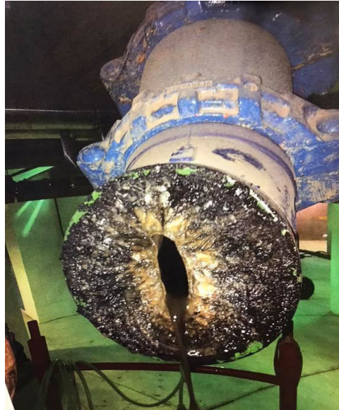
Struvite deposits inside a digester pipe.
