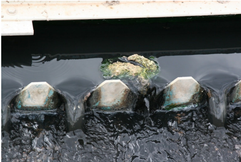
Caked grease (scum) stuck on a primary clarifier weir. Scum is normally scraped off and not sent to the downstream aeration tank.
