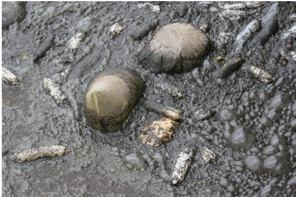
Floating scum in an influent chamber. This debris should be removed and sent to a landfill.
