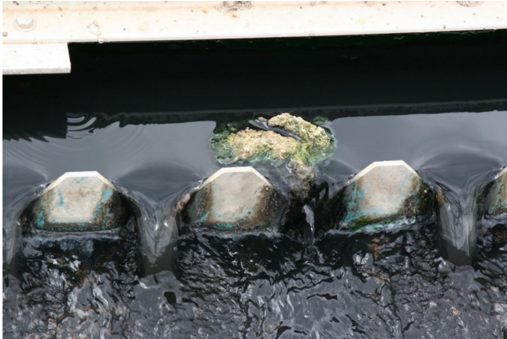
Caked grease (scum) stuck on a primary clarifier weir. Scum is normally scraped off and not sent to the downstream aeration tank.
