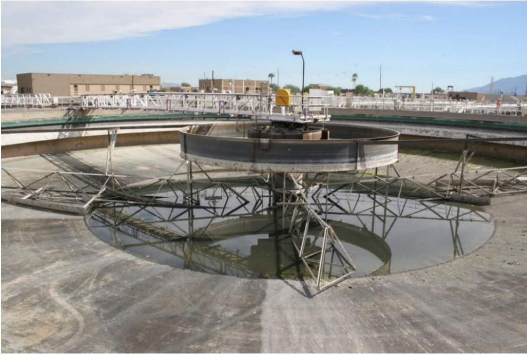
Top photograph, a clarifier's raking mechanism.
