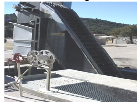
Manual and Mechanical Bar Screens
