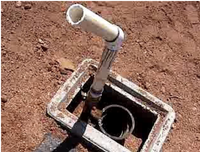
A temporary blow-off at a dead-end line.
