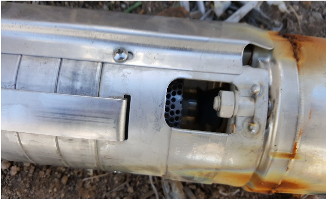
Pump and motor connection.
