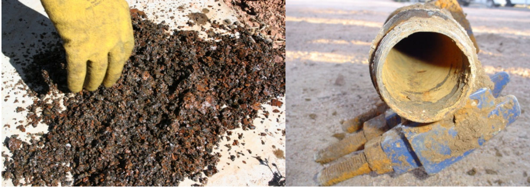
Rust and debris from cleaning a steel main.
