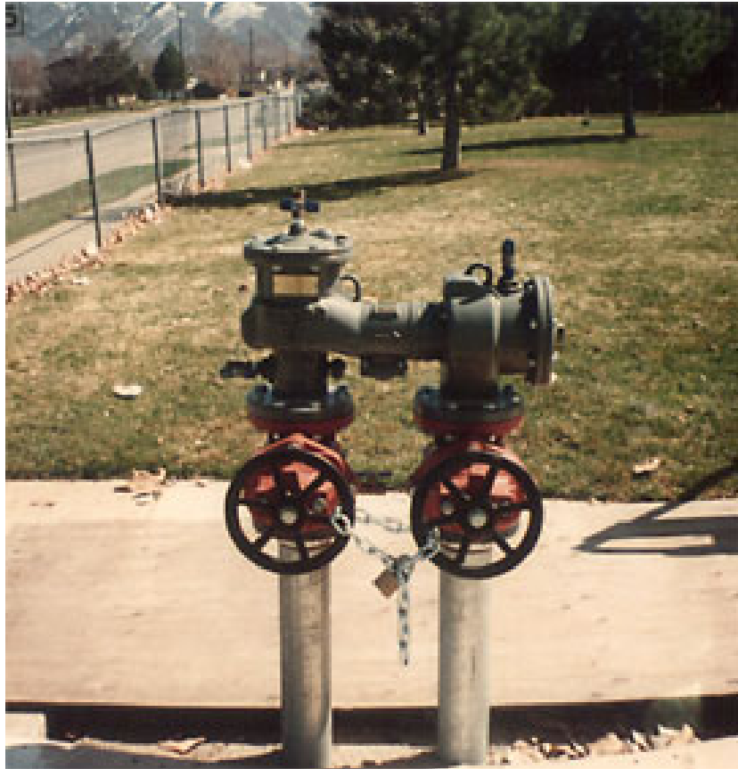
Double Check Backflow Assembly (Notice chain common on OS&Y).
