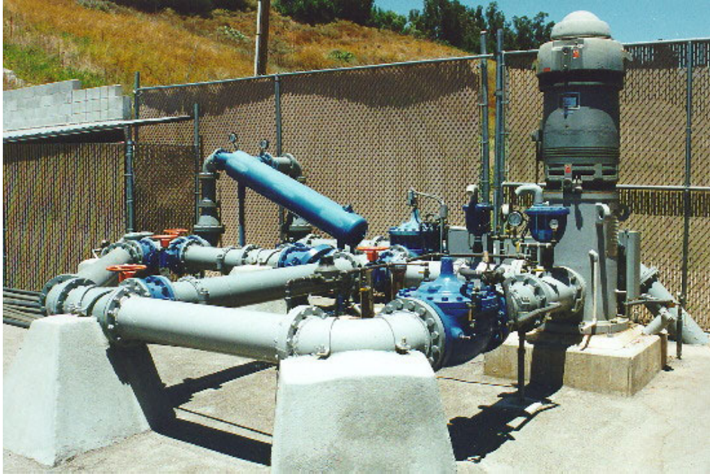
Vertical Turbine Well
