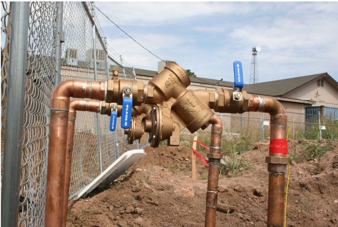
Two brand new RPs ready for inspection.
