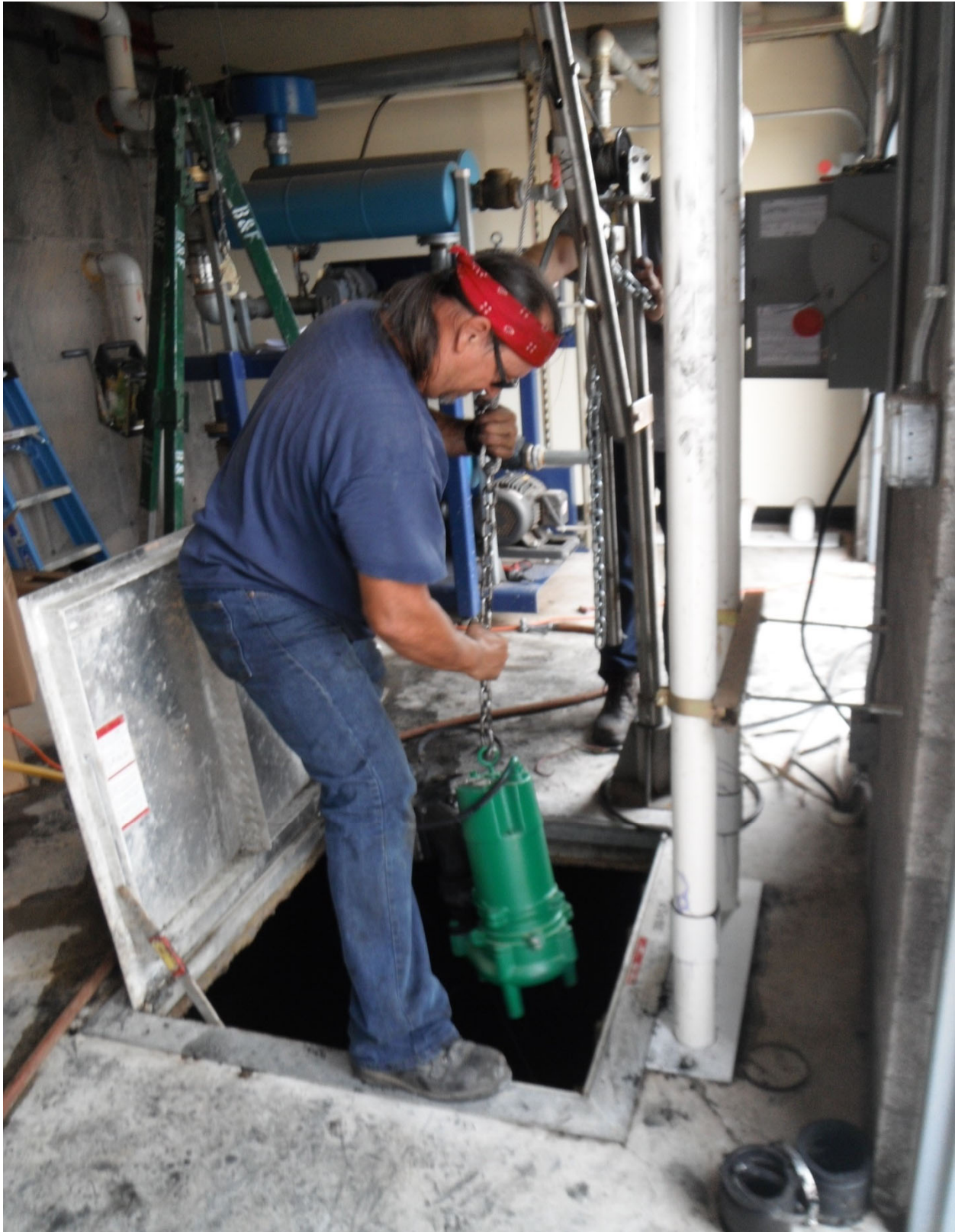
Some of the operating problems you may encounter with centrifugal pumps as an Operator, together with the probable causes, are discussed in the following pages
