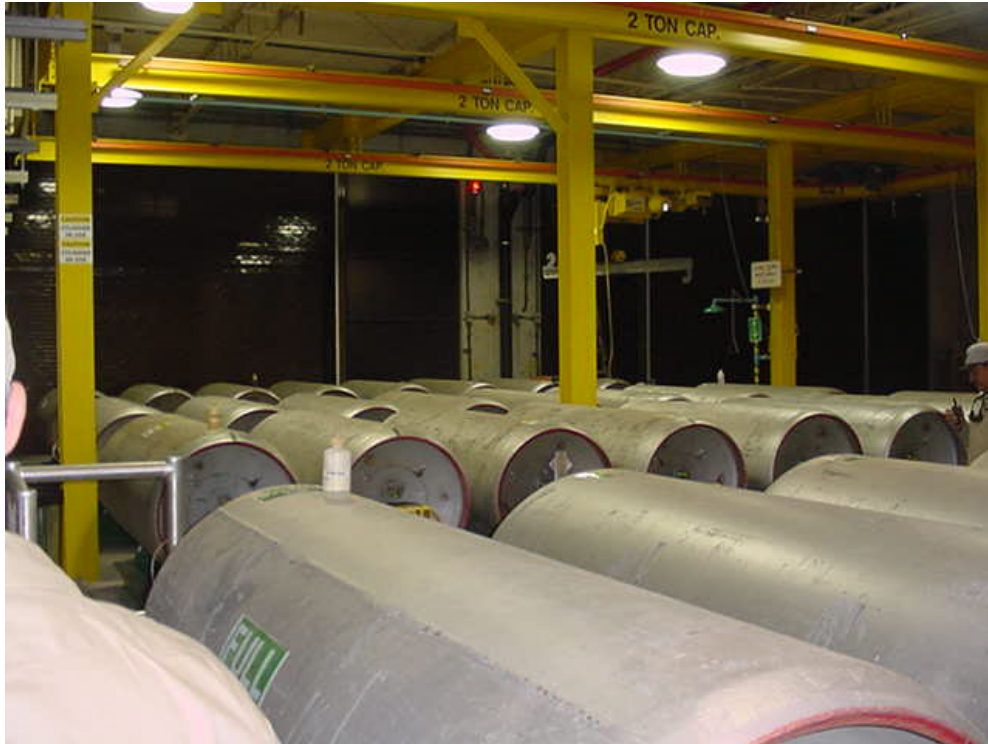
1-ton chlorine gas containers
