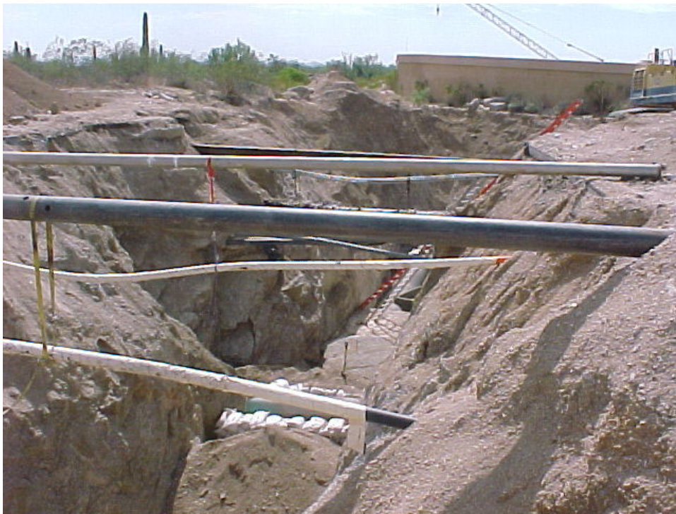
Supporting utilities is mandatory.
