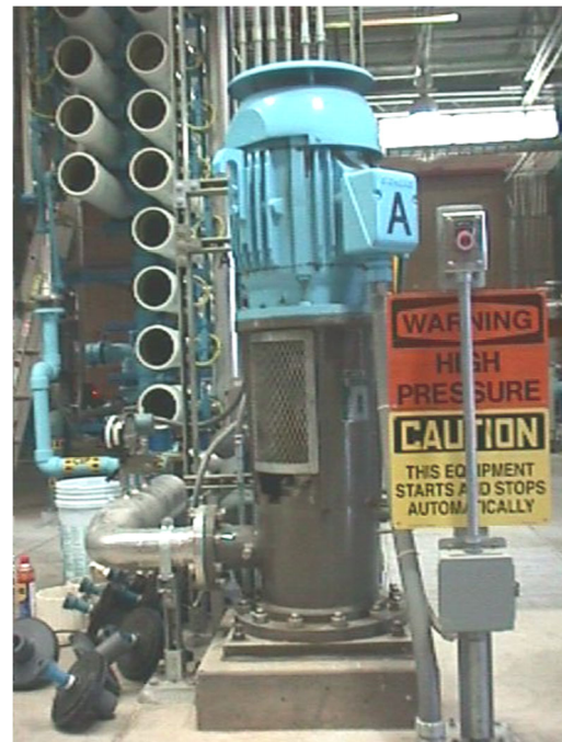
Membrane Filtration System
