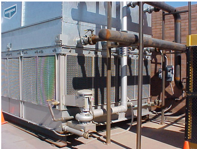
Cooling Tower - A common location for finding a cross-connection.
