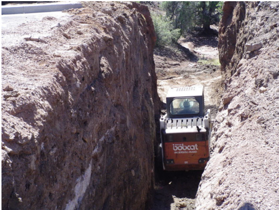
Major OSHA Violation. Do not operate equipment in unprotected trenches. This guy is trying hard to get to Heaven before his time is up.
