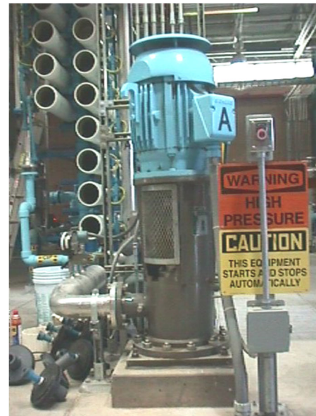
Membrane Filtration System
