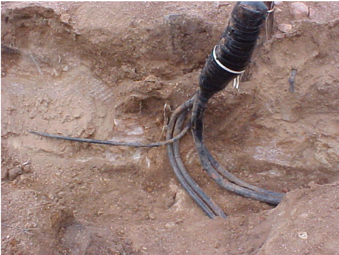
Telephone Cables, nasty to dig around. It's almost as bad as electric lines.
