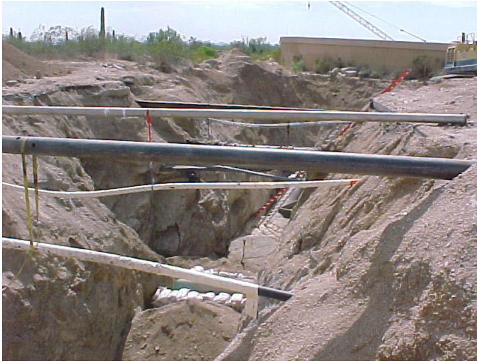
Supporting utilities is mandatory.
