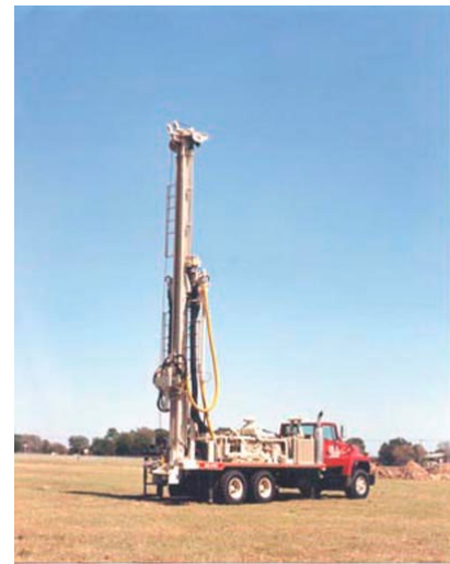
Typical Rotary Rig
