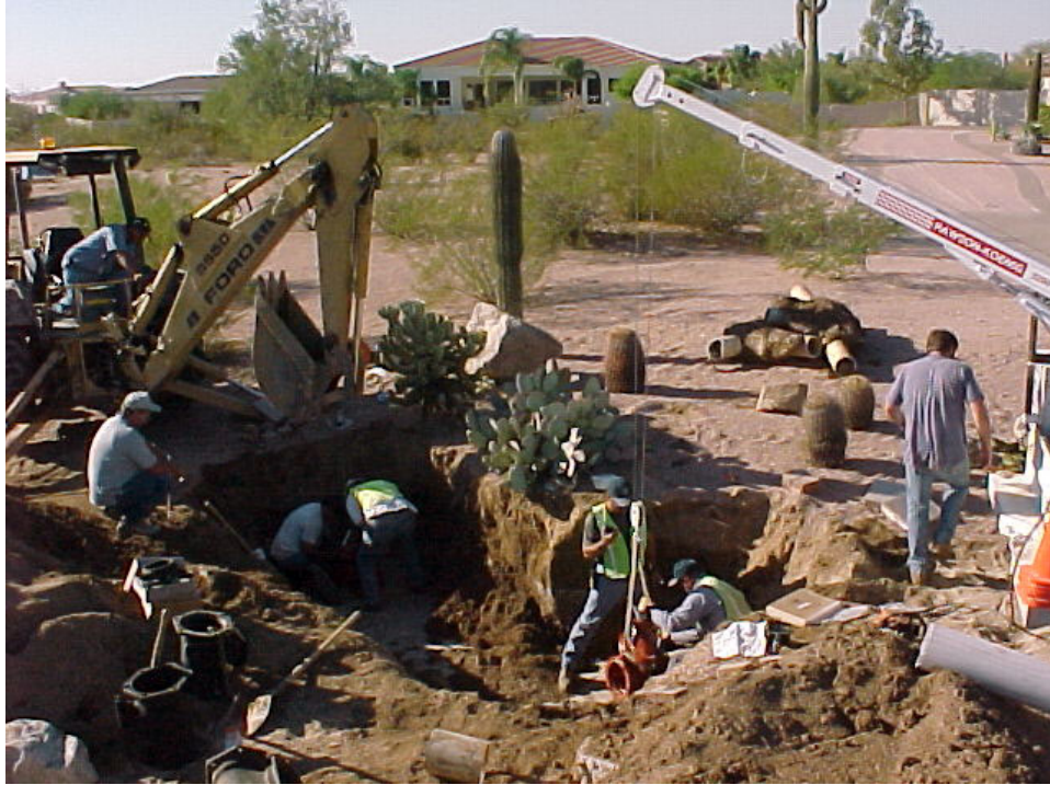
Top photo, two gate valves blew out, you can see the kickers or thrust blocks in the background.
