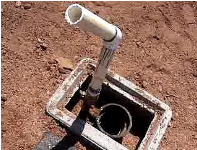
A temporary blow-off at a dead-end line.
