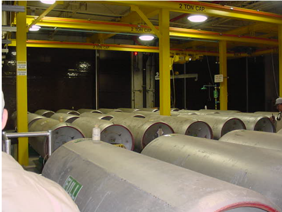
1-ton chlorine gas containers
