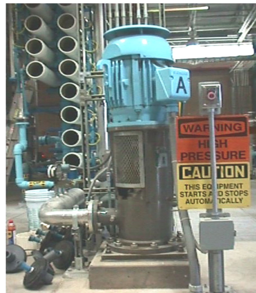
Membrane Filtration System
