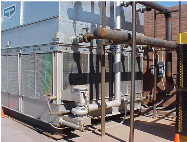
Cooling Tower - A common location for finding a cross-connection.
