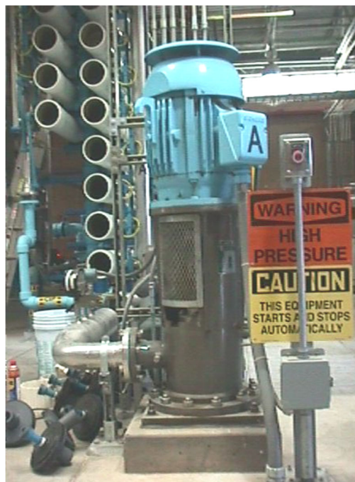
Membrane Filtration System
