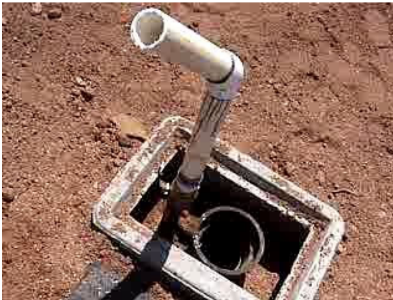
A temporary blow-off at a dead-end line.
