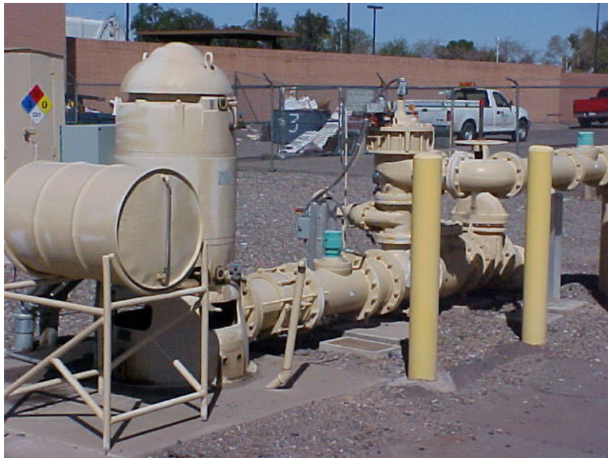
Well with a mineral oil sealed vertical turbine pump
