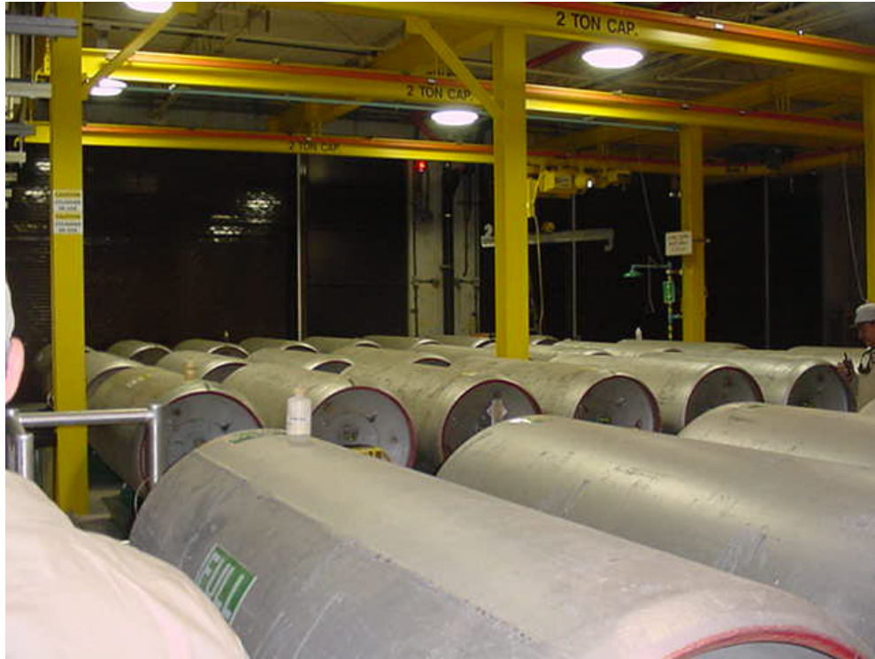
1-ton chlorine gas containers
