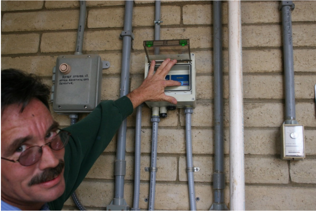
Top photograph, adjusting the chlorine leak alarm sensor. Bottom photograph, chlorine container weight scales.
