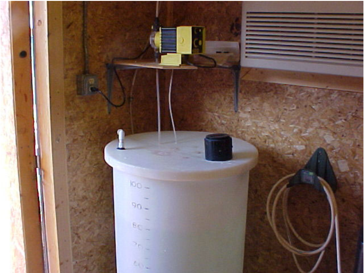
Small chlorine solution tank, normally found on small wells or post-chlorination areas in the distribution system
