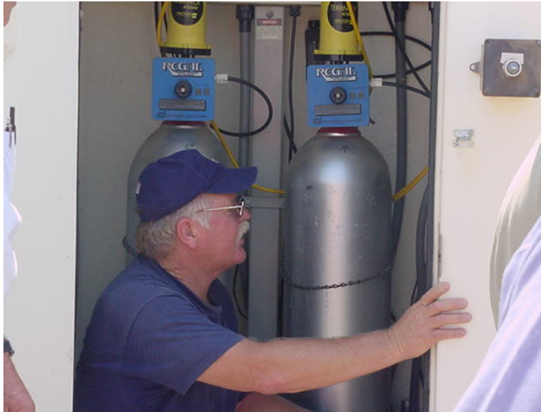
150 pound chlorine cylinder
