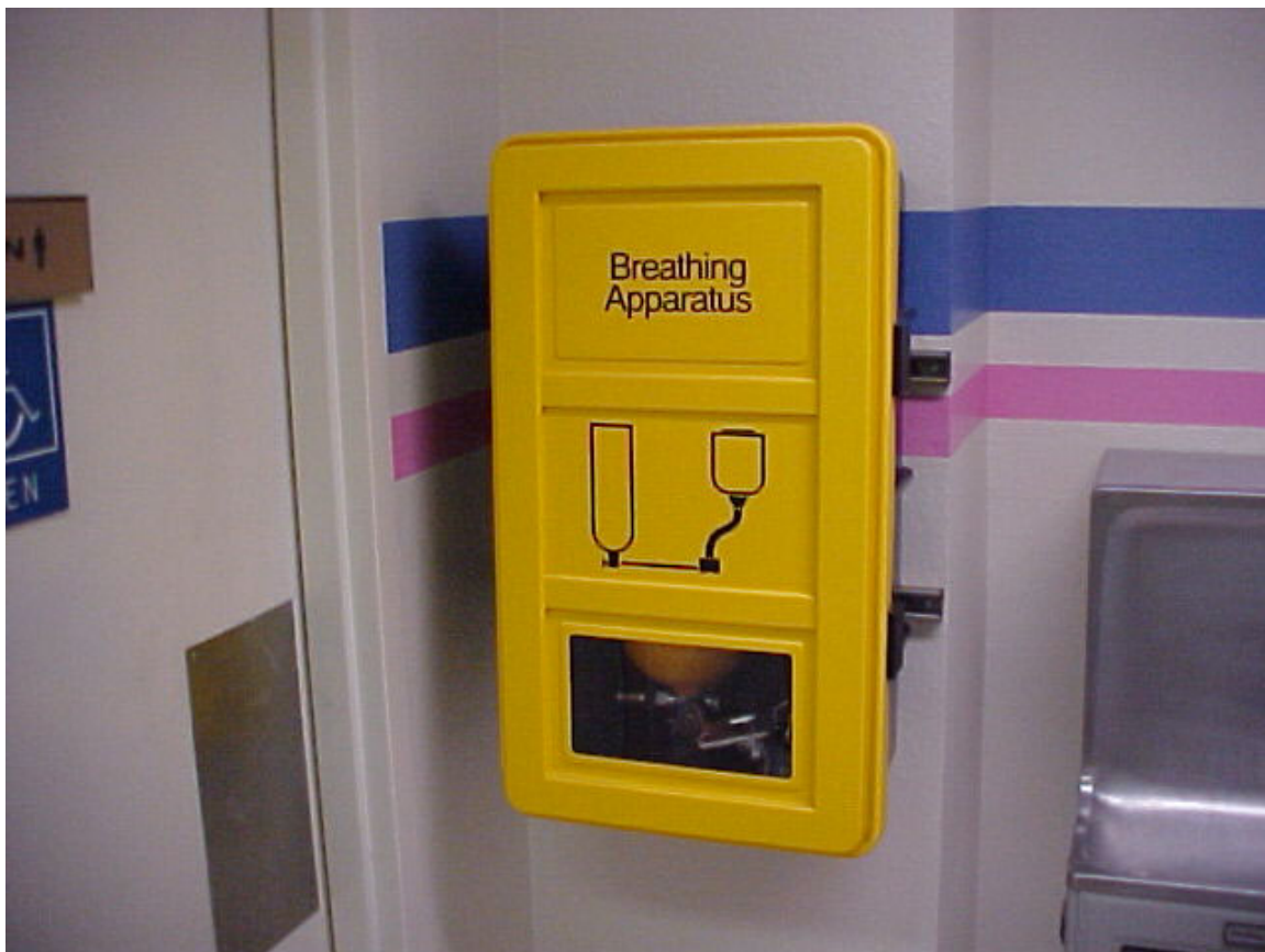
SCBA Storage Box
