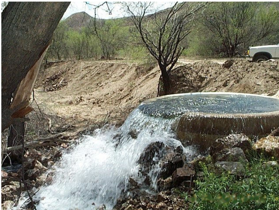
Treated wastewater outfall.
