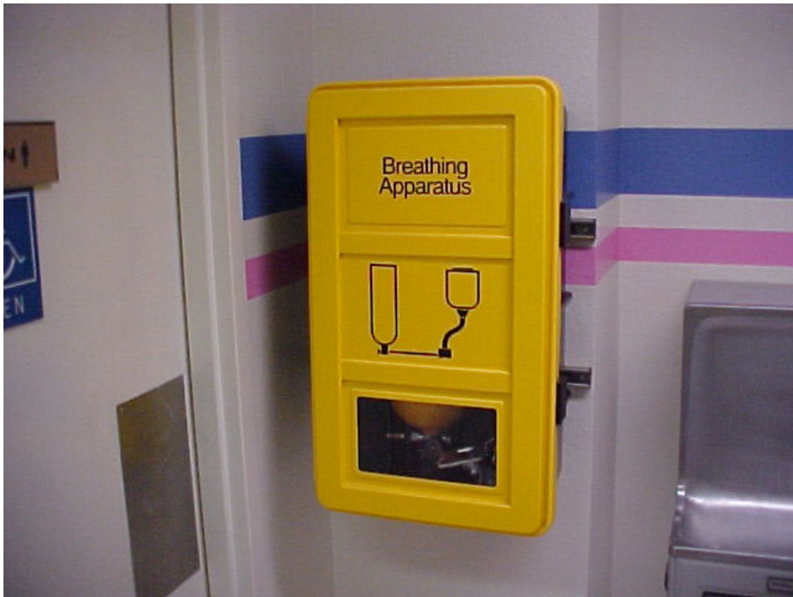
SCBA Storage Box
