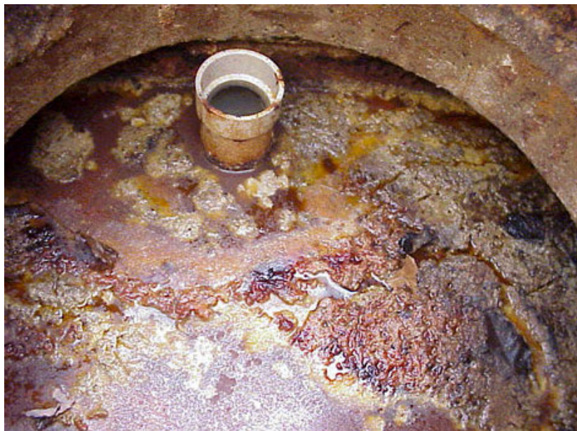
Looking down into a grease interceptor commonly used in a commercial food service operations.
