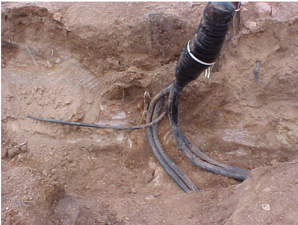
Telephone Cables, difficult to dig around. Not as difficult as electric lines.
