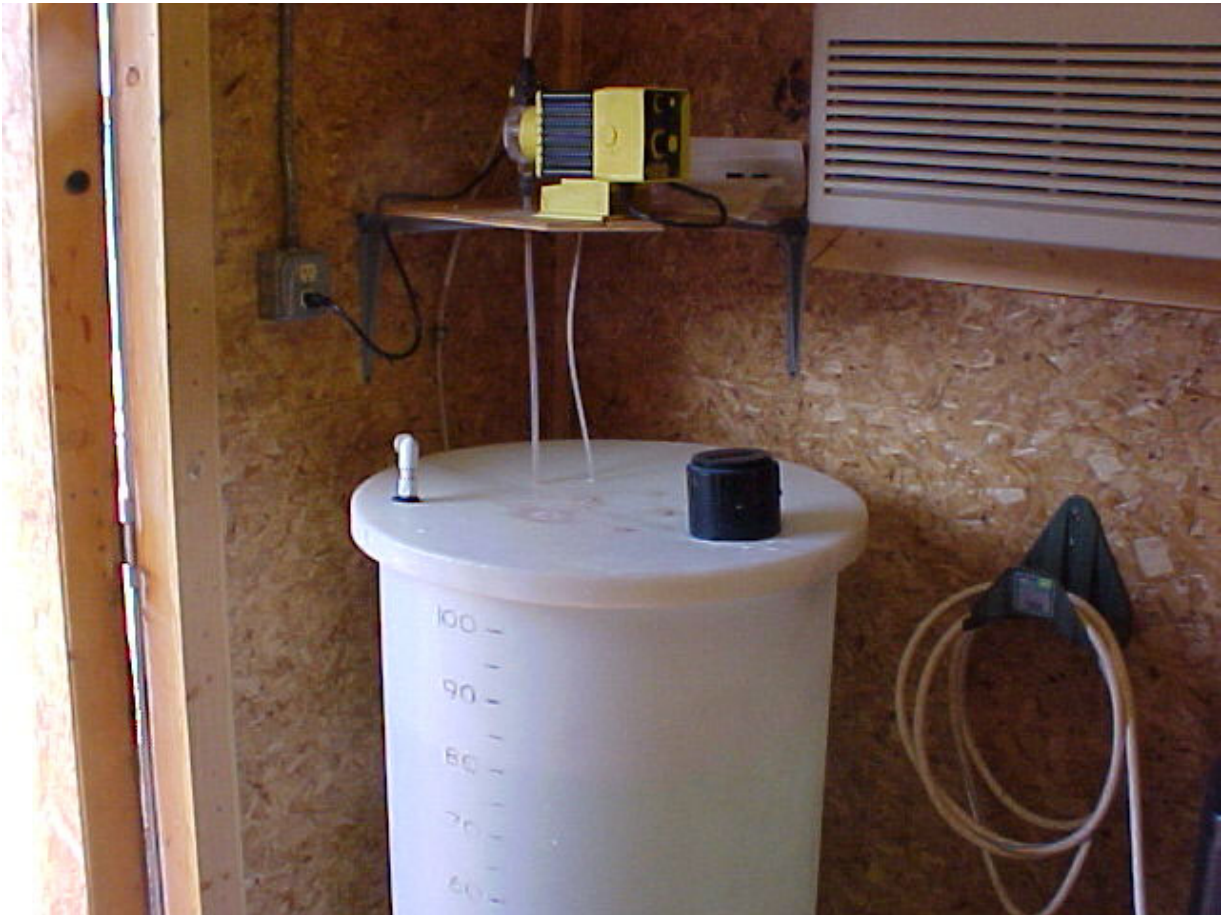
Small chlorine solution tank, normally found on small wells or post-chlorination areas in the distribution system
