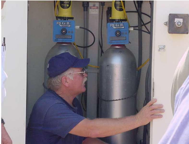
150 pound chlorine cylinder
