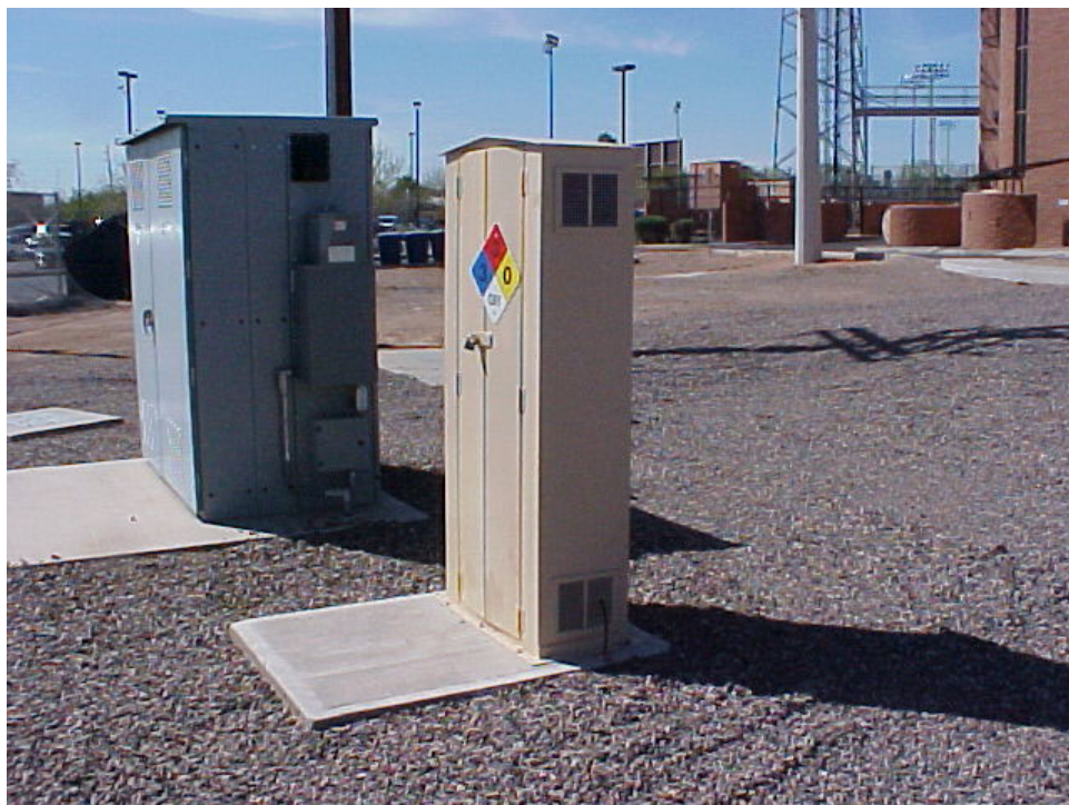
Small chlorine storage shed in the foreground; notice the vents at the bottom and top. The bottom vent will allow the gas to ventilate because \text{Cl}_2 gas is heavier than air.
