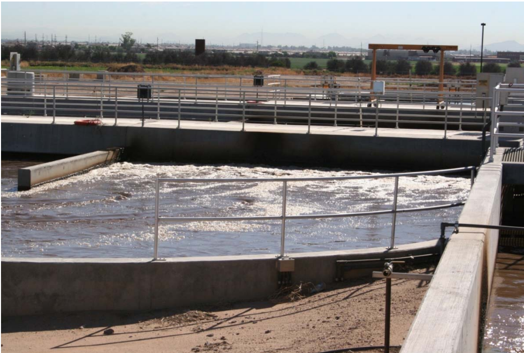
Oxidation ditches are used for nutrient removal.
