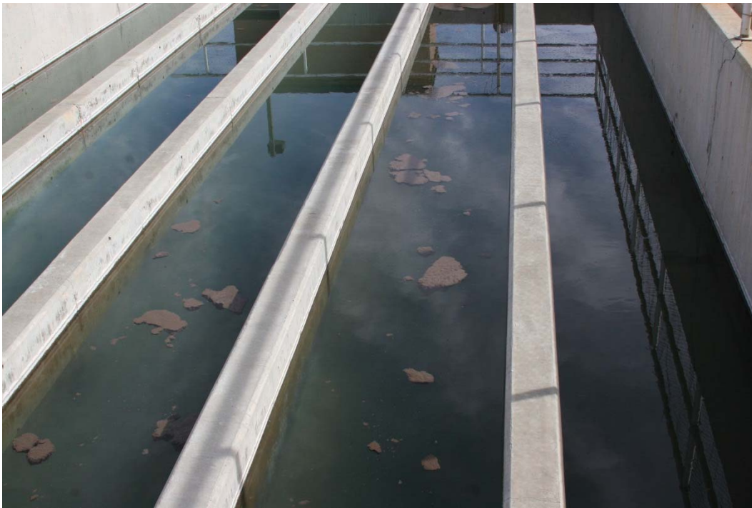
During a slight plant upset, sludge from the filters can be carried over to the chlorine contact channel.
