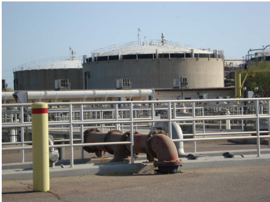
Two massive anaerobic digesters.
