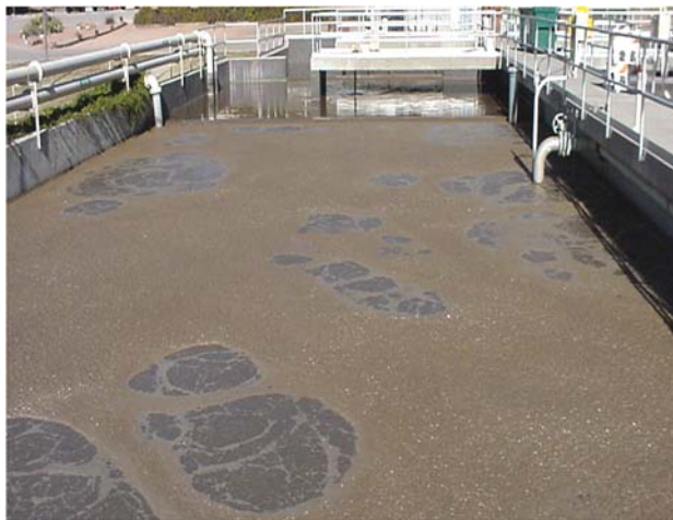
Activated Sludge Aeration Basin, you can tell by the bubbles.
