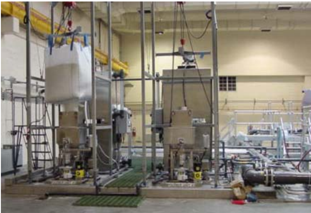
Dry polymer is being added and used for sludge thickening.
