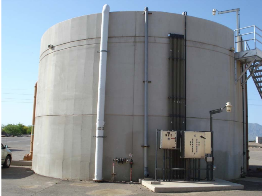
This clarifier is used to thicken sludge prior to the digester, this is not a digester but looks like one. Notice the light on the top for Operators to look inside.
