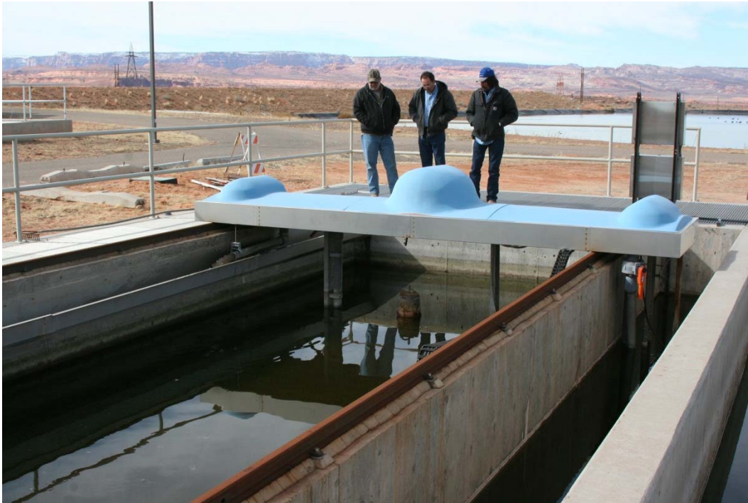
These operators are making sure that the backwash pumps are working for the sand filter.
