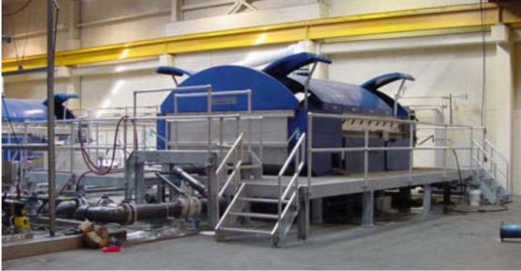
Gravity belt thickeners are often used to remove excess water from sludge.
