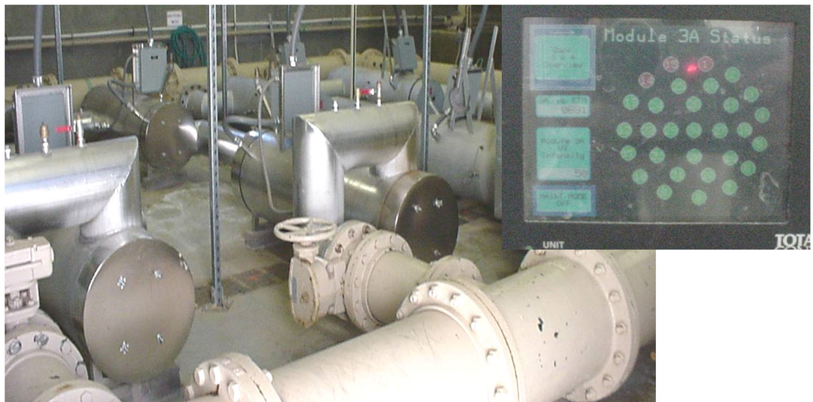
UV Trains and SCADA display.
