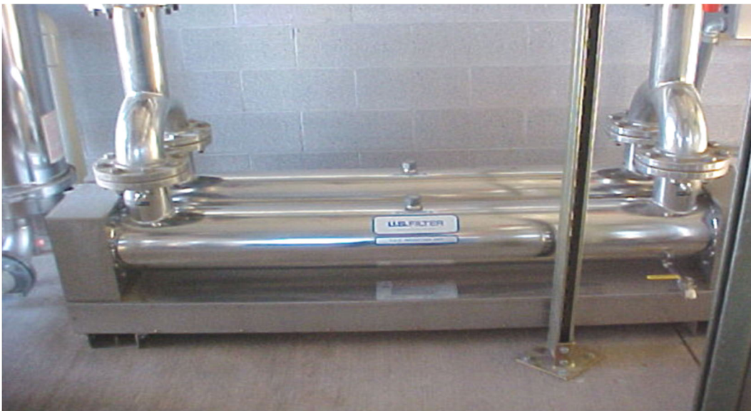
Enclosed lamp system, this one is on wastewater effluent.
