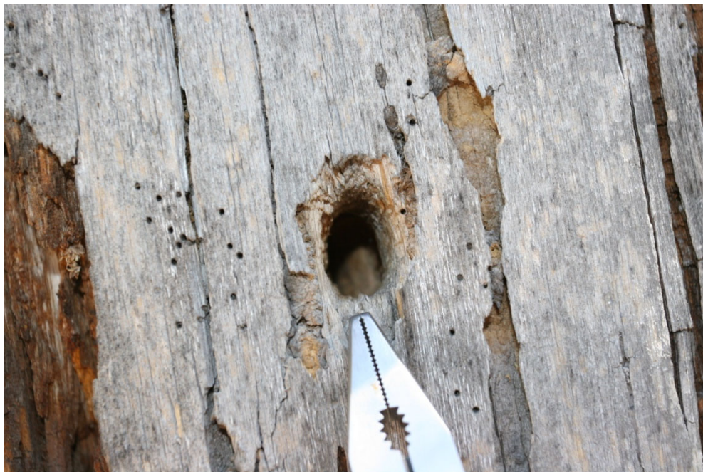
Evidence of Carpenter bee in above photo. Note Woodpeckers do not drill holes longer than their beaks. Woodpeckers are great wood destroyers, even on the sides of houses but the damage is only about 1 inch deep. You will probably go to prison if you try to control a woodpecker. Endangered species act and wildlife regulations are very strict.
