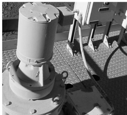
Clarifier Drive Motor
